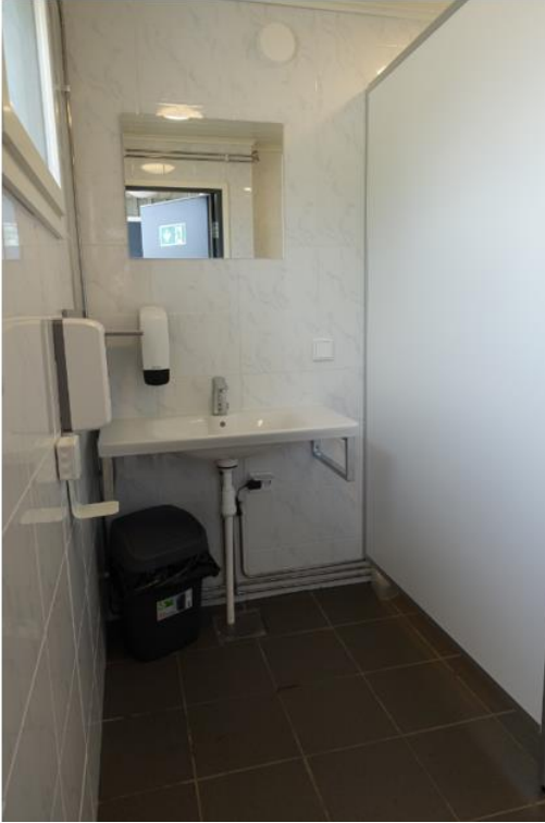
Interior of the new service building. Photo: Metsähallitus / Sanna-Kaisa Juvonen.
