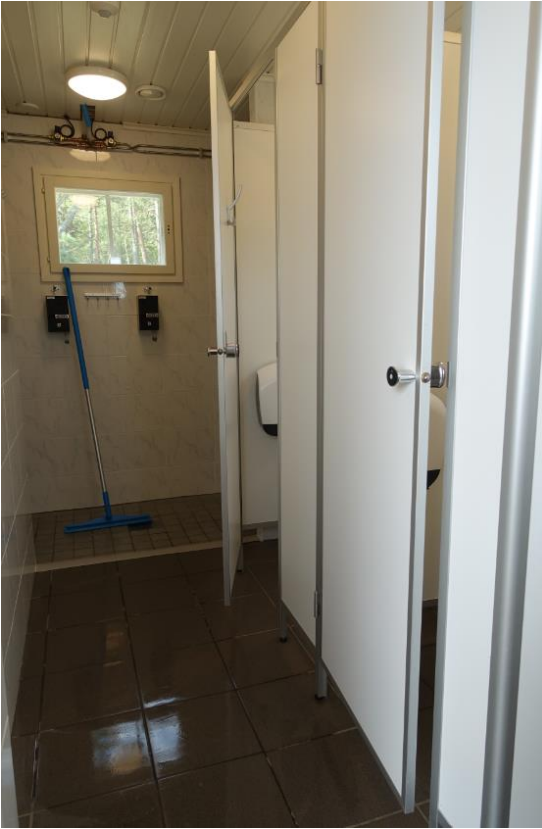
Toilets and shower in the new service building. Photo: Metsähallitus / Sanna-Kaisa Juvonen.
