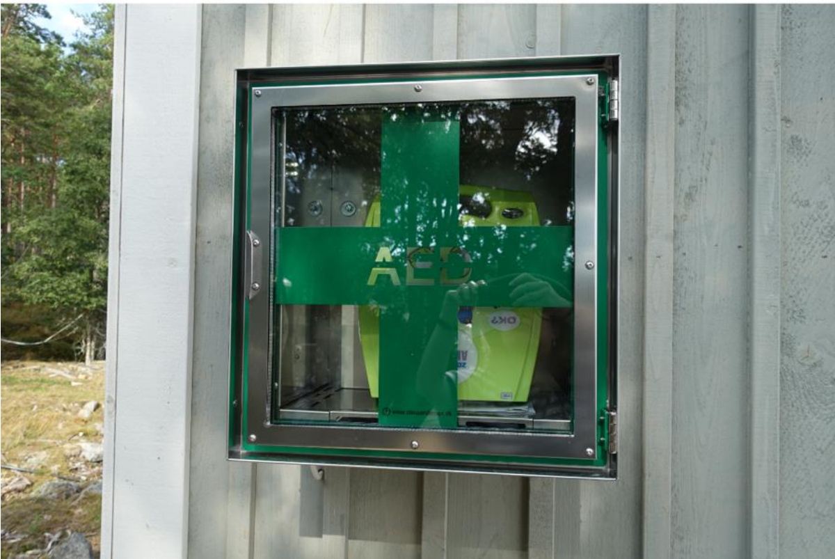
An AED defibrillator unit is installed on the outside wall of the service building. Photo: Metsähallitus / Sanna-Kaisa Juvonen.
