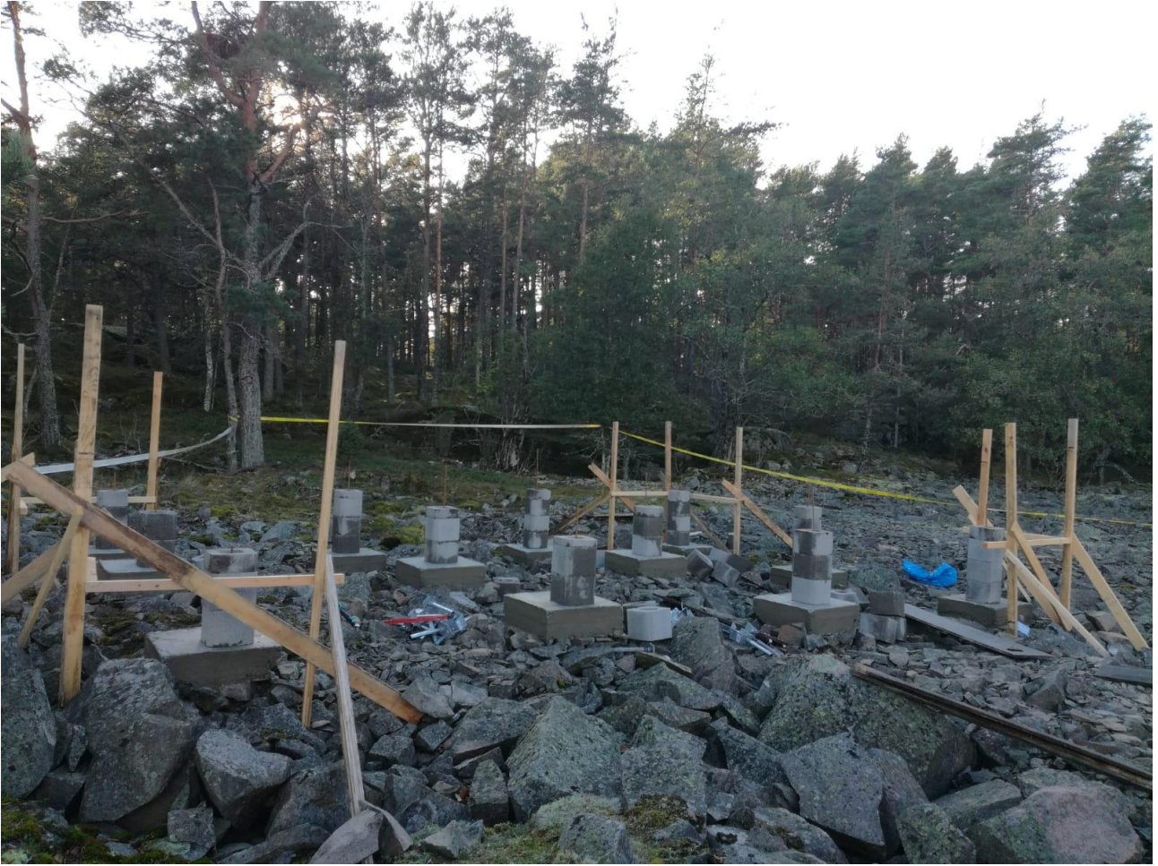
The location of the new service building on Katanpää at the onset of construction work. Photo: Captain's Table.
