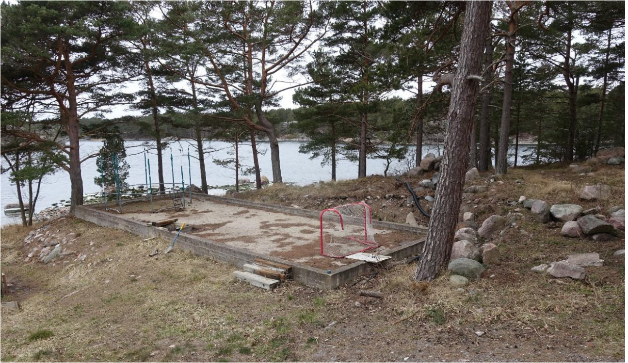
The location of the new service building on Bodö at the onset of the construction work. Photo: Metsähallitus / Sanna-Kaisa Juvonen.
