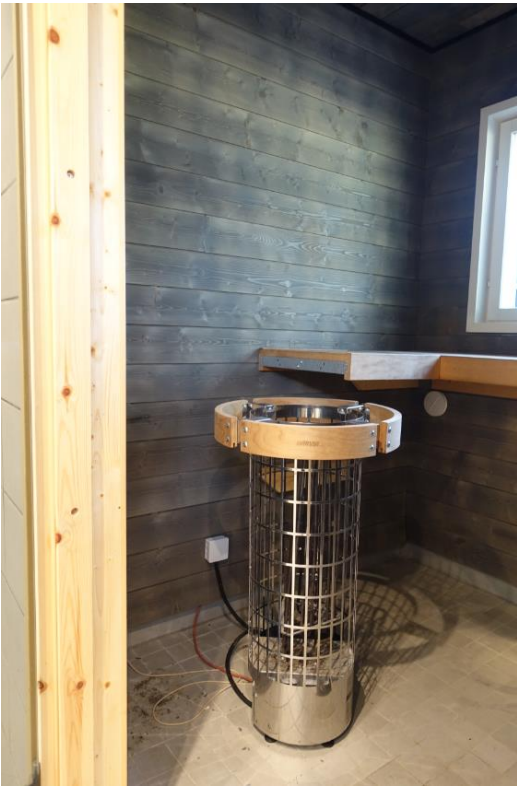
Sauna stove in the sauna of the service building. Photo: Metsähallitus / Sanna-Kaisa Juvonen.
