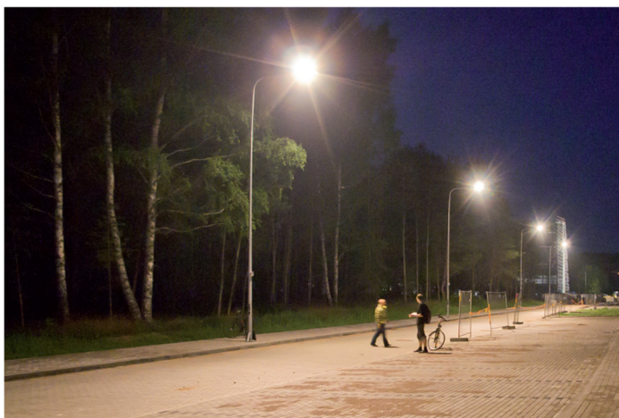
Fig.2.10: Lighting installation at Vilnius University campus
