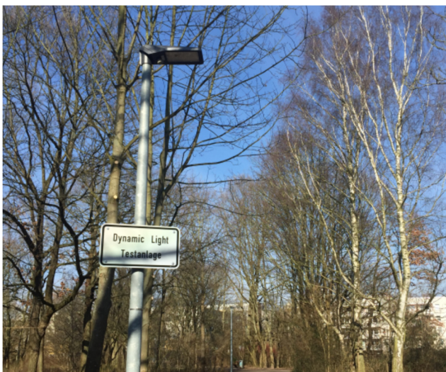
Figure 3.7: Luminaires of test implementation
