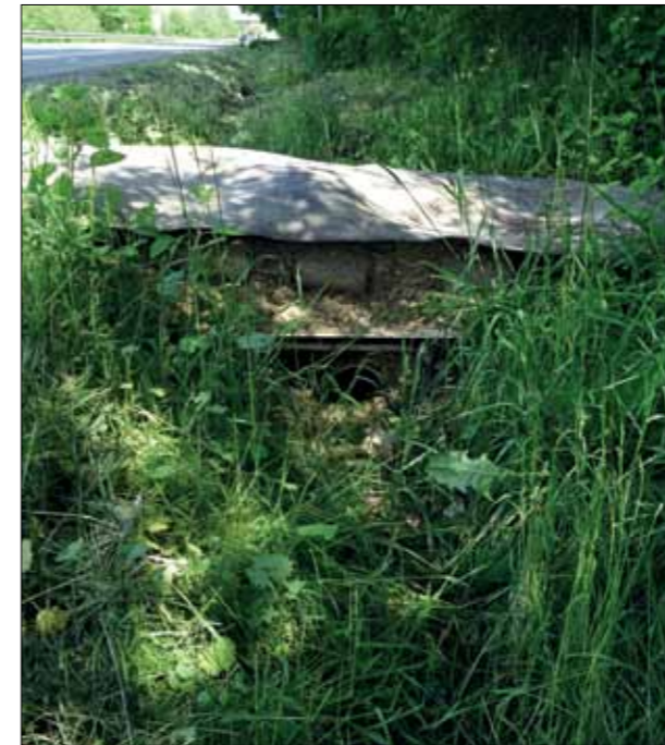
Figure 4.11 Swale degraded by an irresistibly formed bridge for the transition. Photo: B. Vojvodíková
