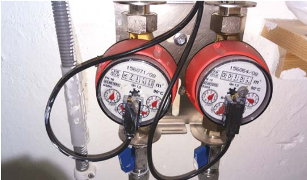
Figure: Smart meters installed in the apartments
