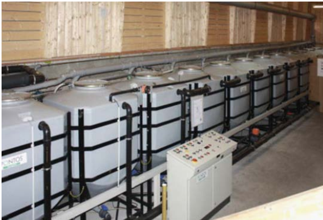
Figure 12: A multi-stage moving bed biofilm reactor (MBBR) for greywater recycling in a residential building (Photo: E. Nolde).
