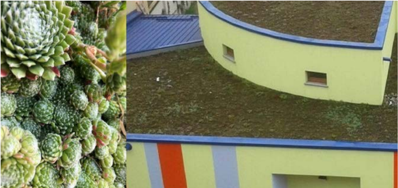
Figure 14: Extensive green roof - sedum, sempervivum - Paguro Children playhouse, Torino (Photo: A. Aires).
