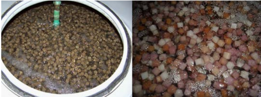
Figure 13: Aerated moving-bed biofilm reactor (MBBR) (left) and foam cubes as carrier media (Photo: E. Nolde).
