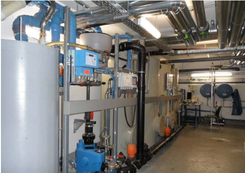
Figure 24: The greywater recycling system including heat recovery from greywater in the cellar of the building.
