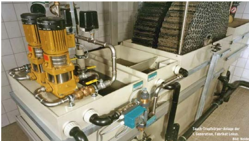
Figure 11: Rotating biological contactors (RBC) in a multi-storey building. First-generation system for greywater recycling from 1995 (Photo: E. Nolde).
