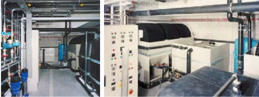
Figure 28: The greywater recycling system with the 6 RBC modules and the post-sedimentation tank.
