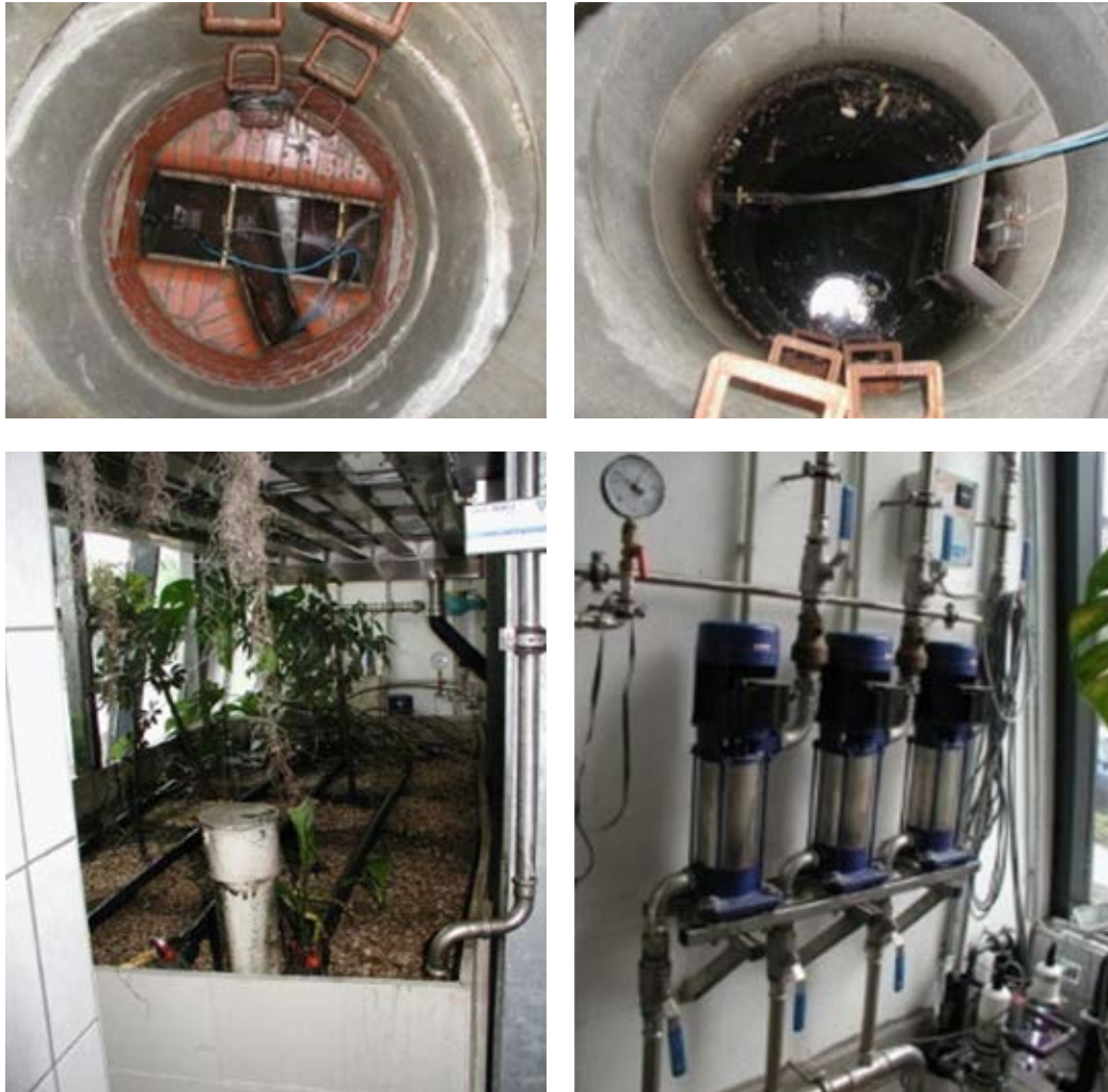
Figure 47: Rainwater sewer with switch diversion (above) and planted soil filter inside the building (below).
