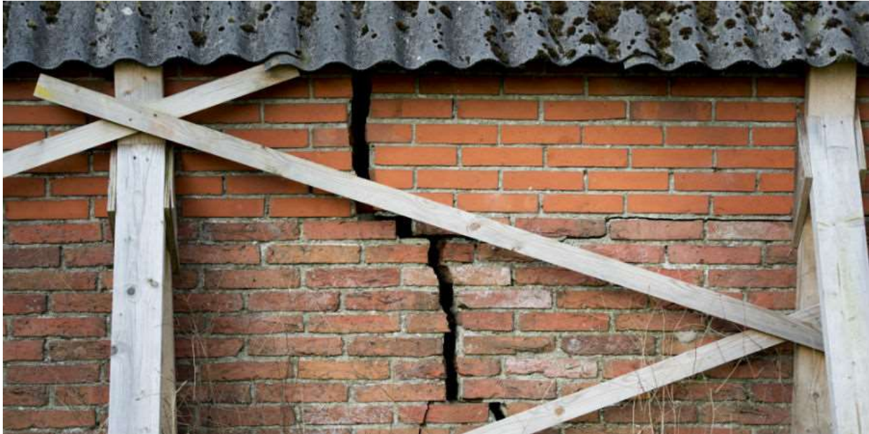
Damage caused by earthquakes due to the extraction of gas.
