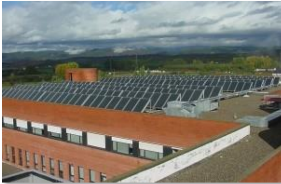
Solar thermal panels on an hospital roof in Ponferrada - León, Castilla y León (EREN)
