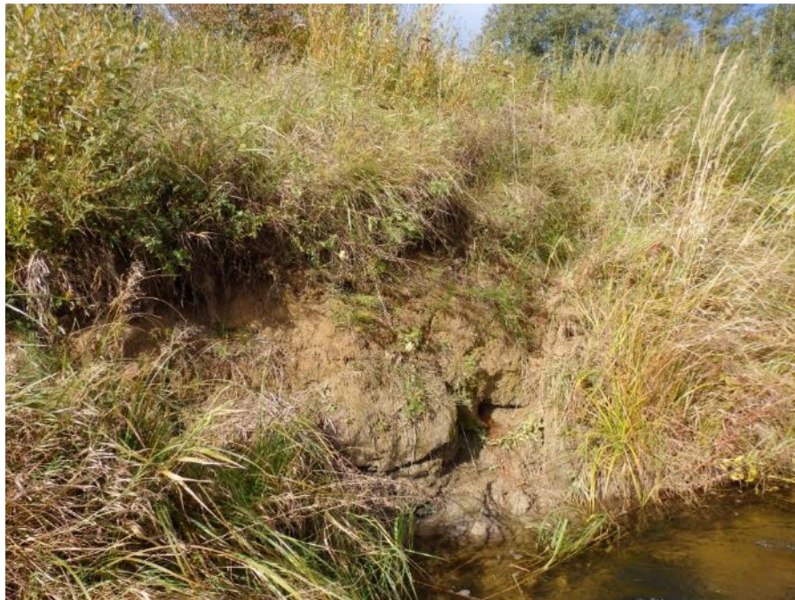
Figure 28 River eroding activity, signs of sufusion (Photo L. Gr̃nberga, 2019)
