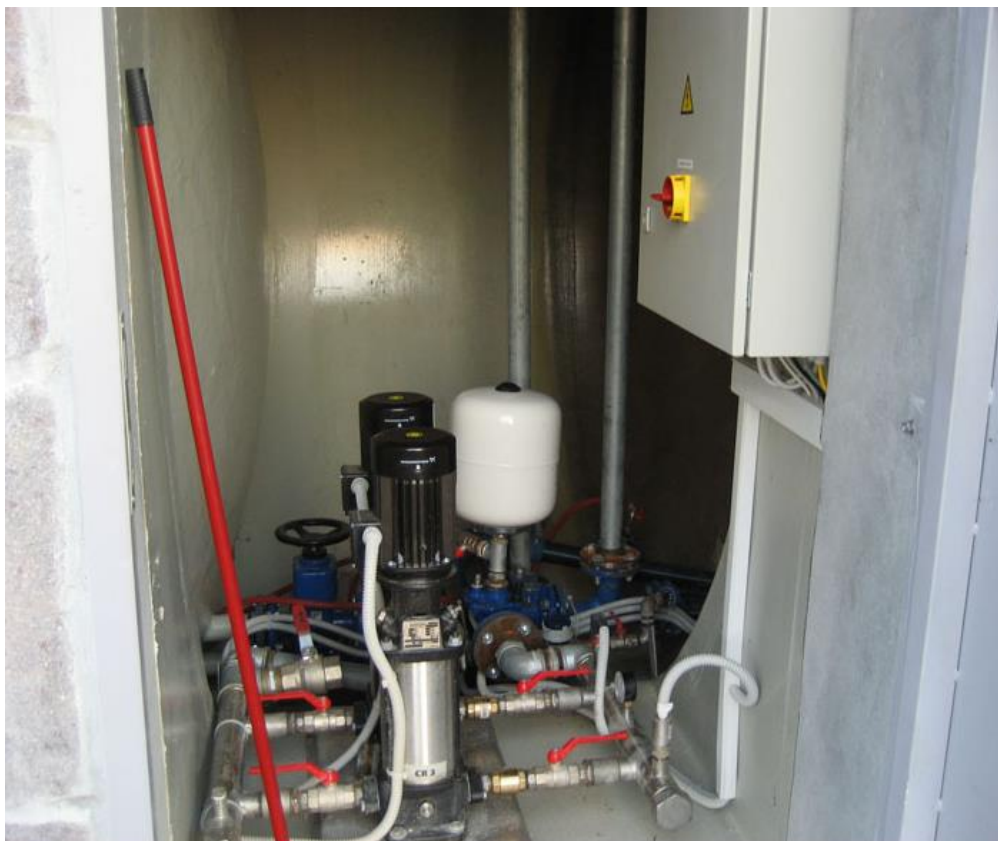
Figure 5. Photo of the pumping station.
