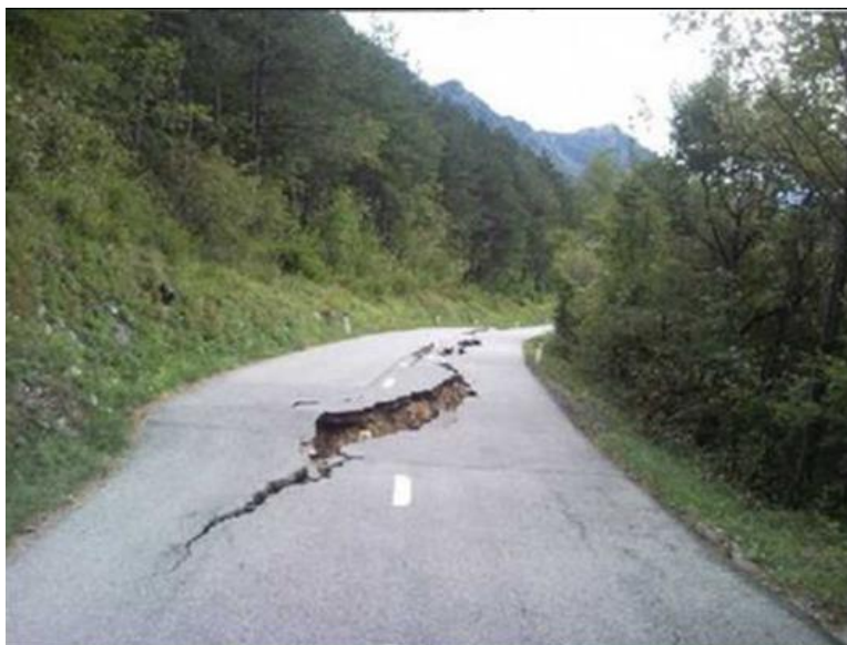
Figure 8. Landslide on the access road to the water reservoir 1
