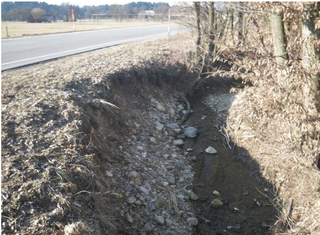
Figure 6. Example of the erosion exposed pipe
