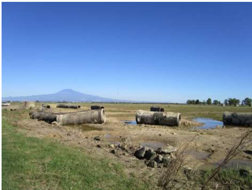
Figure 2. A water pipeline damaged after a flood in Catania Plain, Oct. 2018. Source: DPC Archive.
