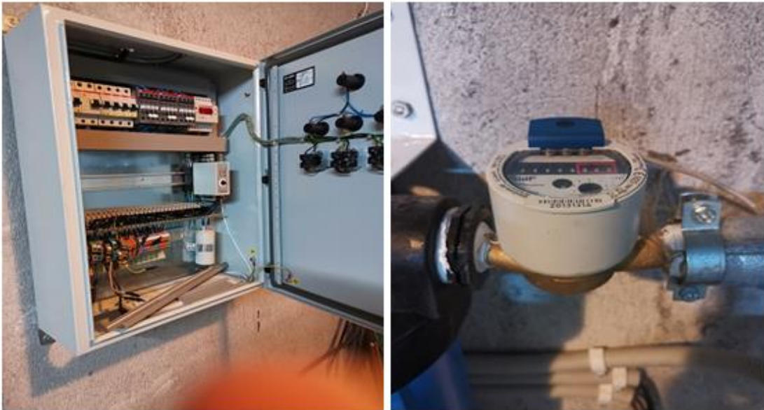
Image 5: Switchboard and flowmeter
