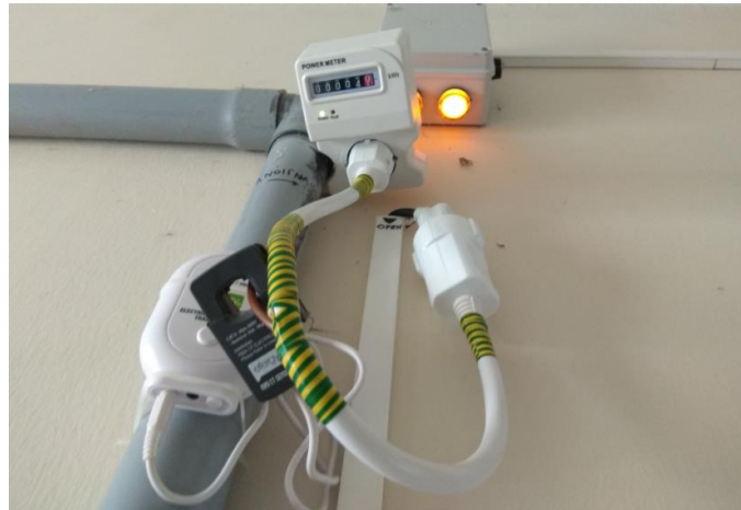
Figure 14. Installation of analogue and Wi-Fi digital power consumption measurement device (Pump C1). The isolated current phase of the cable to achieve power consumption measurement inductively is clearly depicted.
