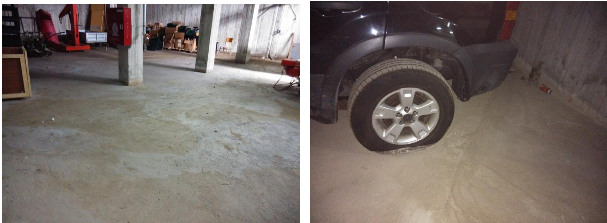
Figure 4. Discolored floor slab indicates the previous presence of stagnant water (left), whereas thick layer of dirt/soil is visible near objects that were not moved after flooding events (right).
