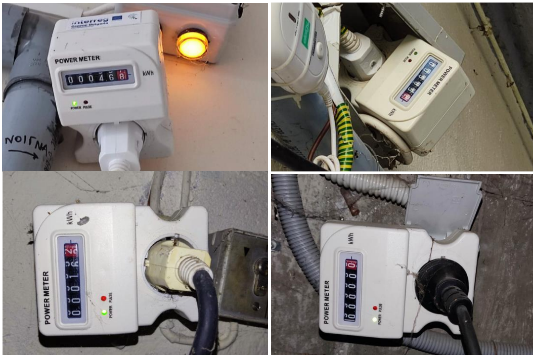
Figure 15. Power consumption measurements of existing water pumps in a) Building C (Pump C1 on the top-left and Pump C2 on the top-right) and (b) Building B (Pump B3 on the bottom-left and Pump B1 on the bottom-right), (photos taken on 11/02/2022).
