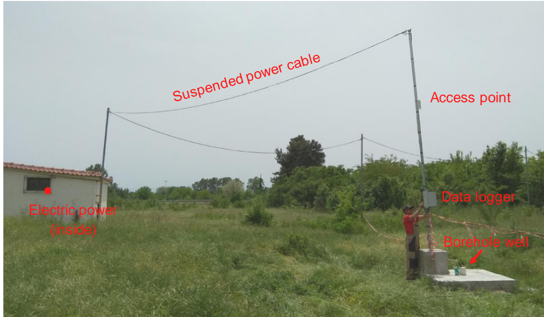
Figure 26. A 6m steel pipe is anchored to the concrete base. The water level monitoring device is installed on this steel pole and transmits measurements via Wi-Fi.
