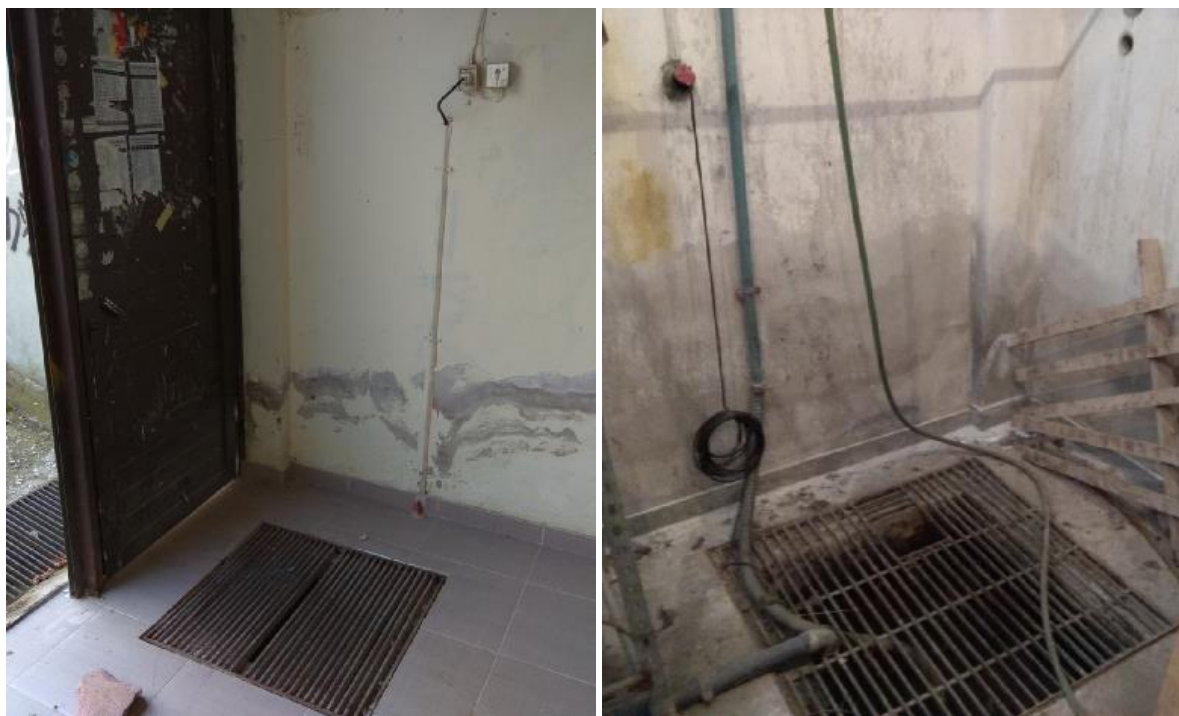
Figure 7. Water pumps are located inside manhole size wells, near power supply, at basement level (Building B - number 6 of Figure 6).
