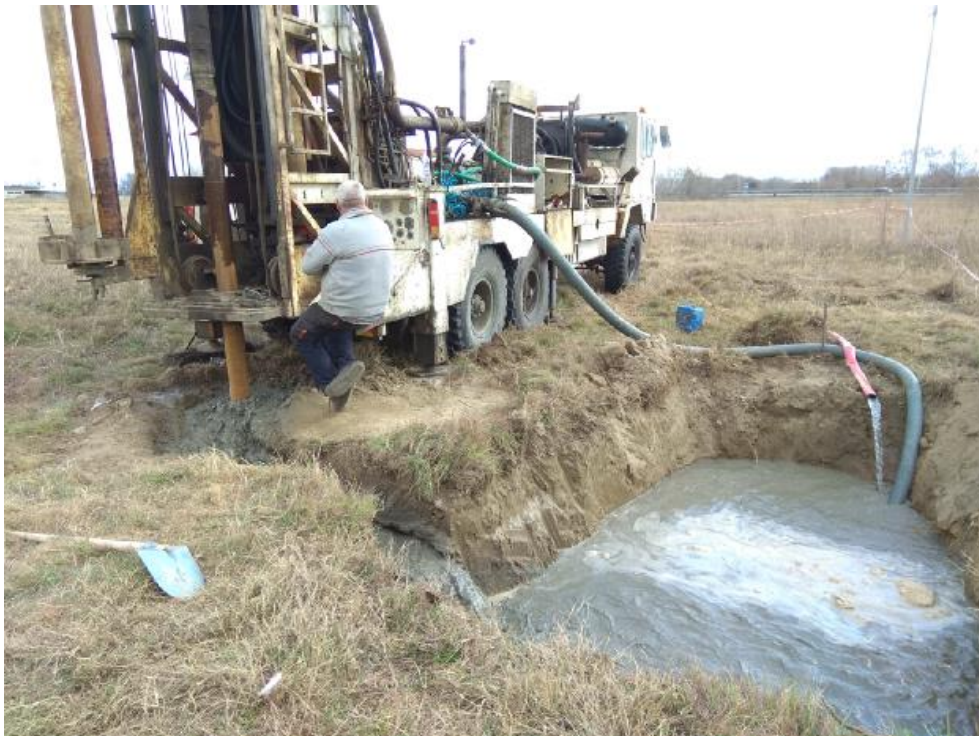
Figure 23. Drilling procedure (the two-fold use of the excavation to provide water and accept the drilling materials can be observed)
