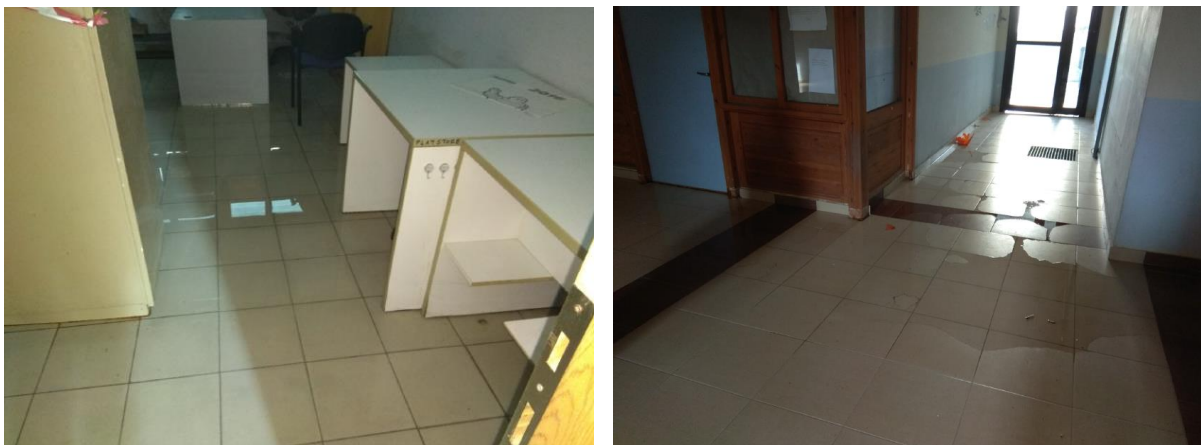
Figure 5. Flooding of teaching rooms or laboratories may disrupt educational procedure and endanger expensive equipment.
