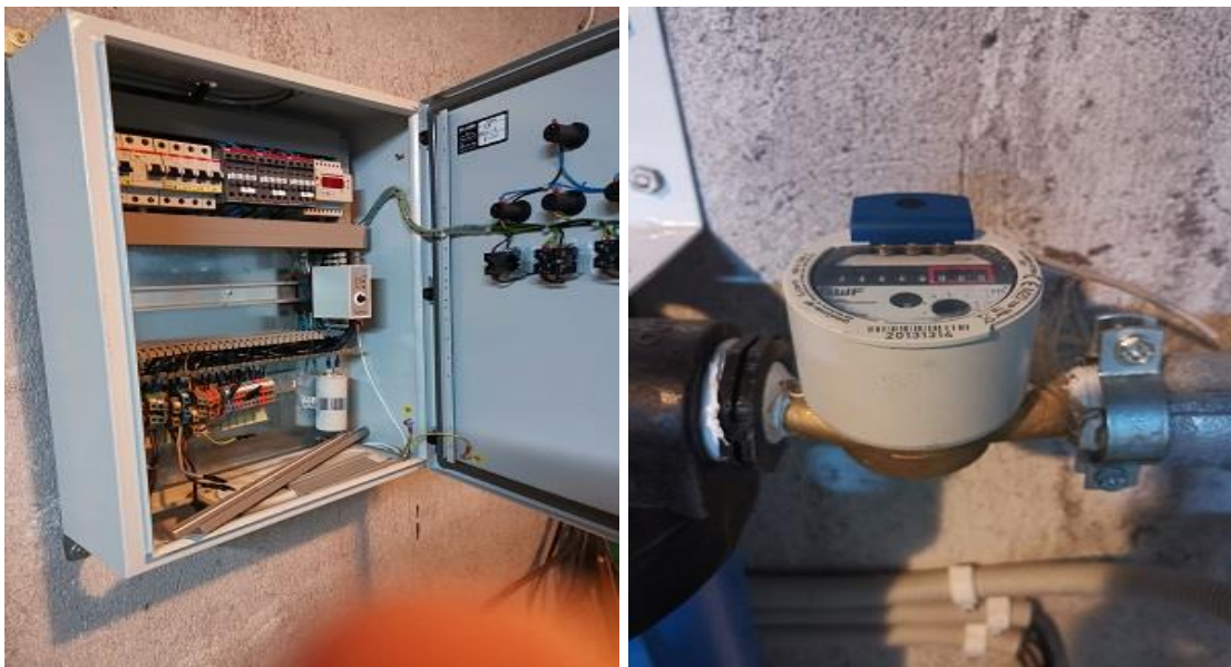
Image 3.5 Switchboard and flowmeter
