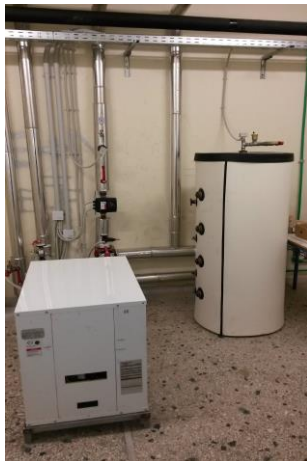
Figure 2. Geothermal heat pump (1 st Gymnasium of Pilea)
