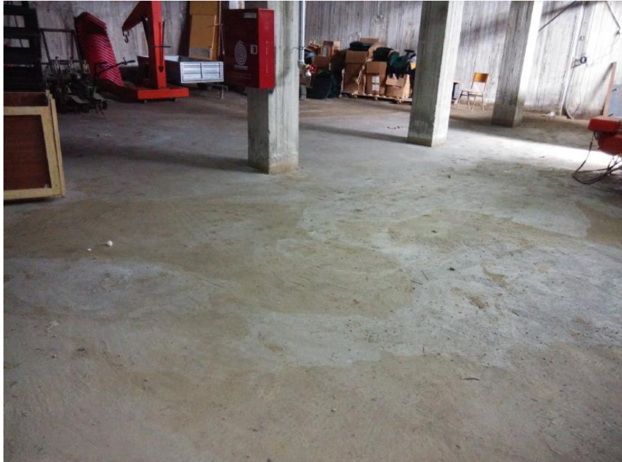
Figure 9. Discolored floor slab indicates the previous presence of stagnant water.
