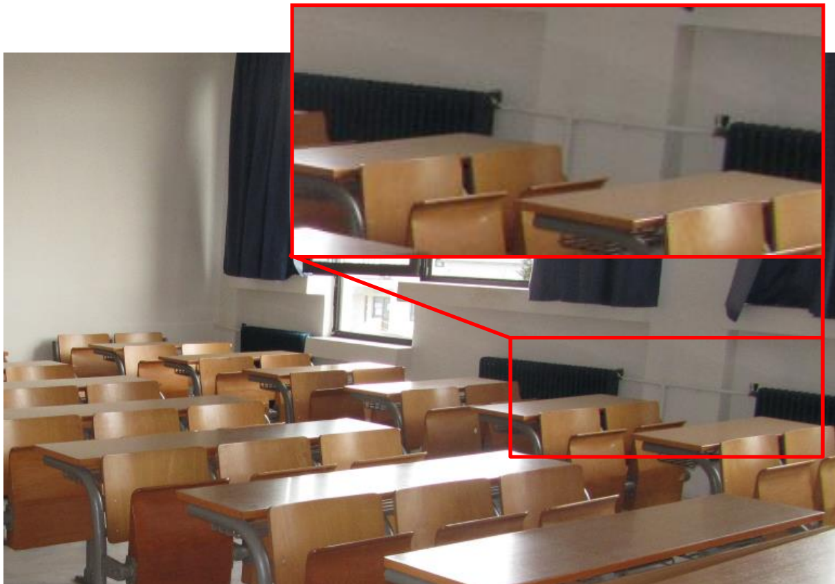
Figure 22. Radiators as part of the central heating system of Building B (piping is visible).
