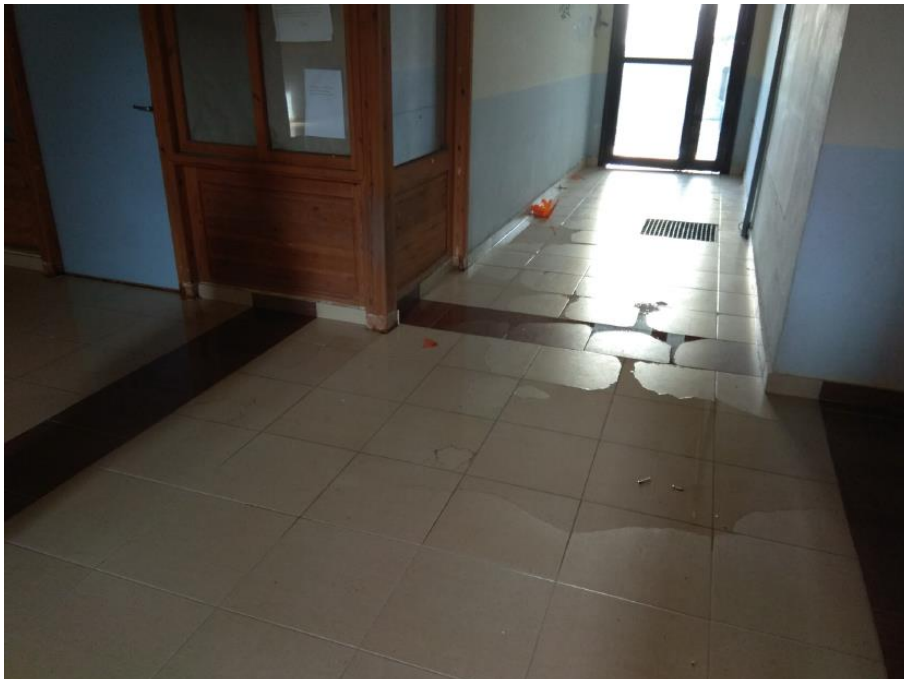
Figure 12. Flooding at basement level (hallway of building).
