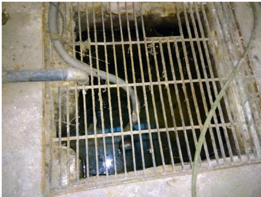
Figure 15. Water table level depth is only a few centimeters below the basement level (Building B - number 6 of Figure 13).
