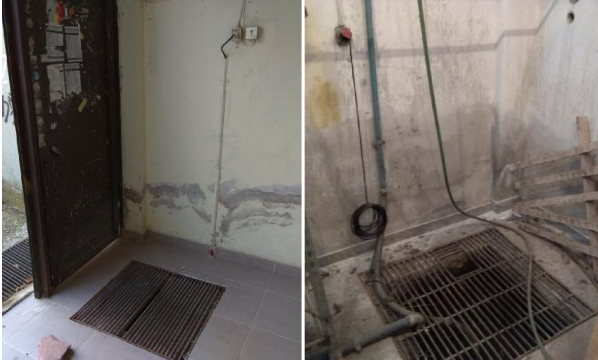
Figure 14. Water pumps are located inside manhole size wells, near power supply, at basement level (Building B - number 6 of Figure 13).
