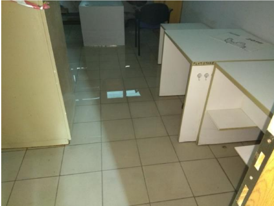
Figure 11. Flooding of teaching rooms or laboratories may disrupt educational procedure and endanger expensive equipment.
