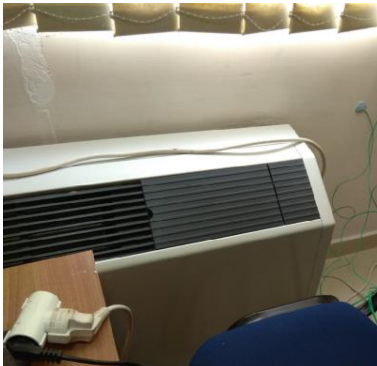
Figure 24. Fan coil units for heating of the 3 rd floor offices.
