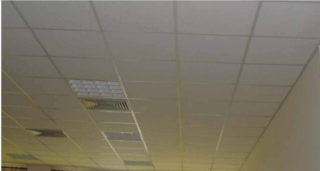
Figure 23. Central air distribution system for classrooms of the 3 rd floor.
