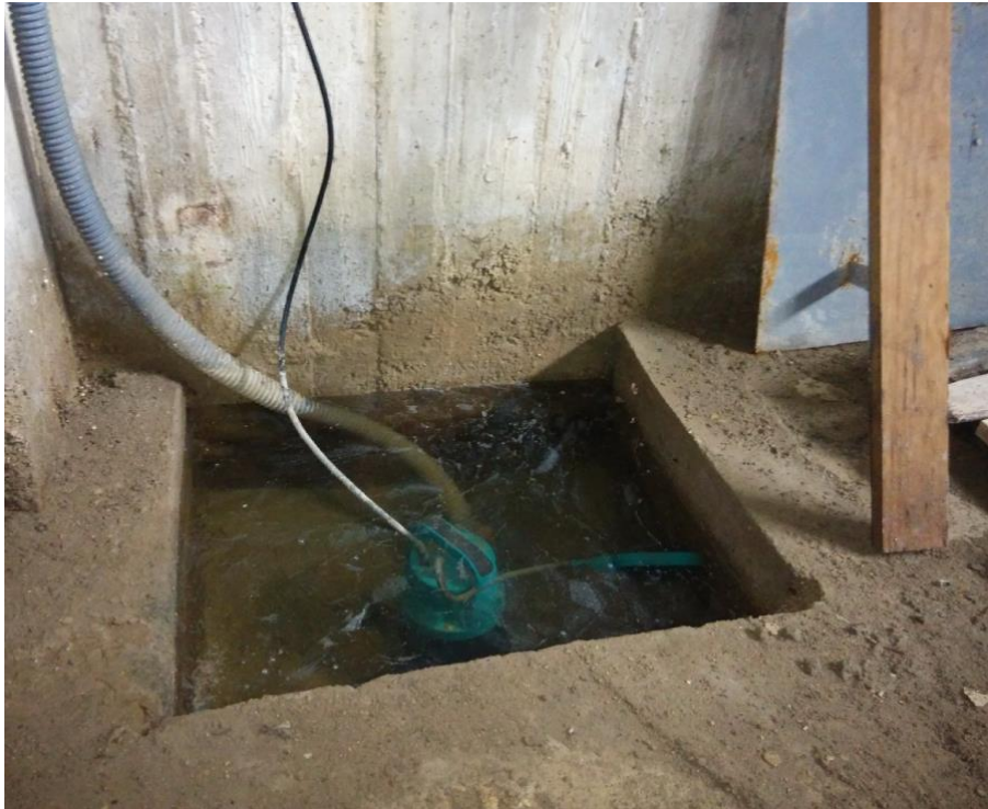
Figure 16. Water table level depth is only a few centimeters below the basement level (Ceremony Hall basement - building number 12 of Figure 13).
