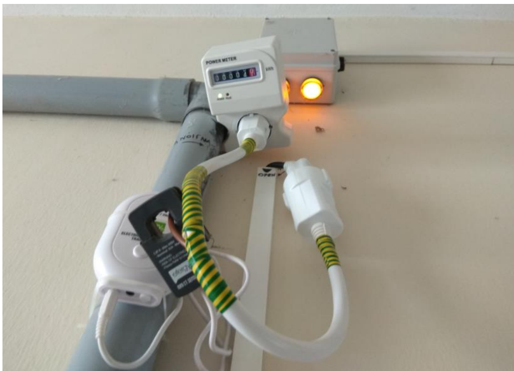
Figure 23. Installation of analogue and Wi-Fi digital power consumption measurement device (Pump C1). The isolated current phase of the cable to achieve power consumption measurement inductively is clearly depicted.
