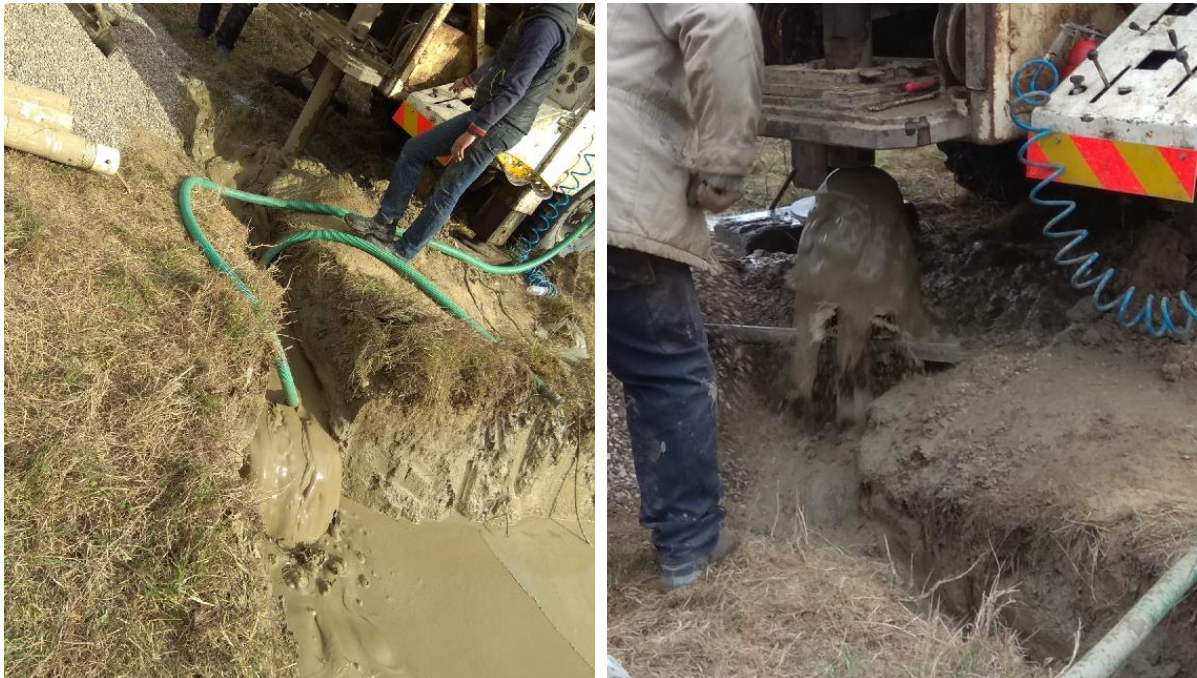
Figure 38. Bentonite material to assist in the drilling process (left side) and removal of bentonite when the gravel pack is placed inside the well surrounding the pipes (right side)
