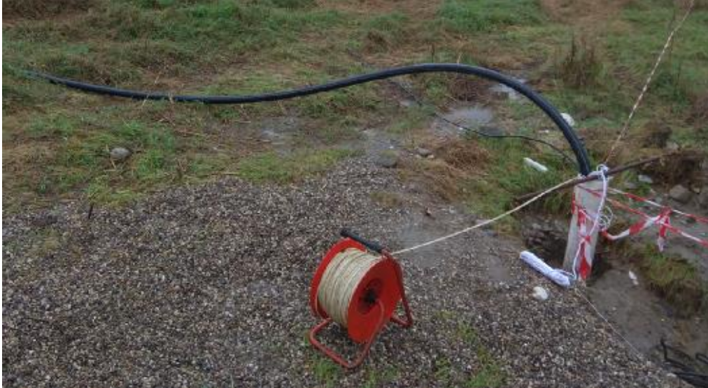
Figure 40. Water pumping during flow testing and simultaneous aquifer depth measurement
