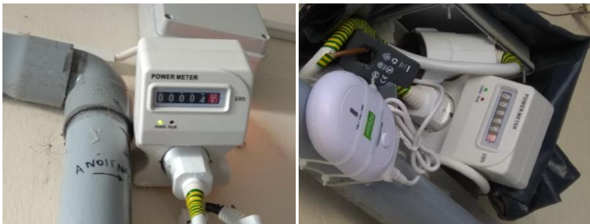
Figure 24. Indicative power consumption measurements of existing water pumps in Building C (Pump C1 on the left and Pump C2 on the right, photo taken on 17/05/2019).
