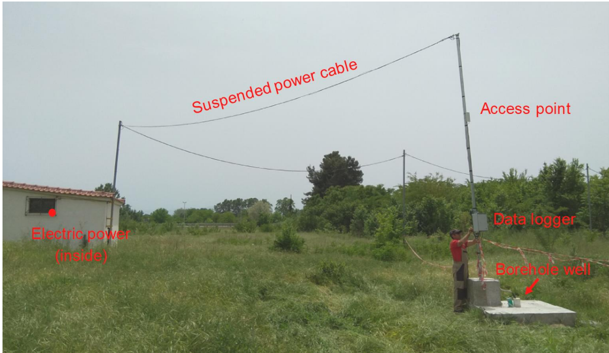
Figure 46. Installation of water level measurement device
