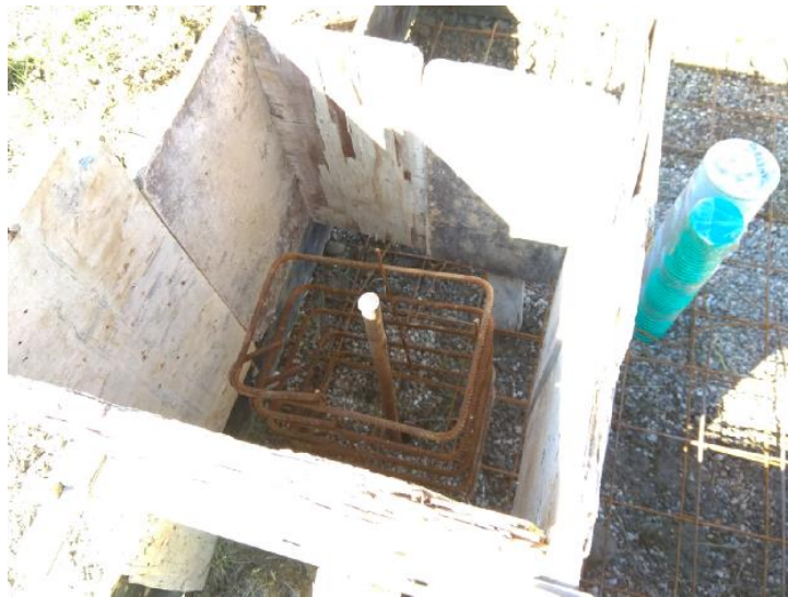
Figure 42. Reinforcement bars of the concrete base and placement of access pipe for future gravel supplement (if required)
