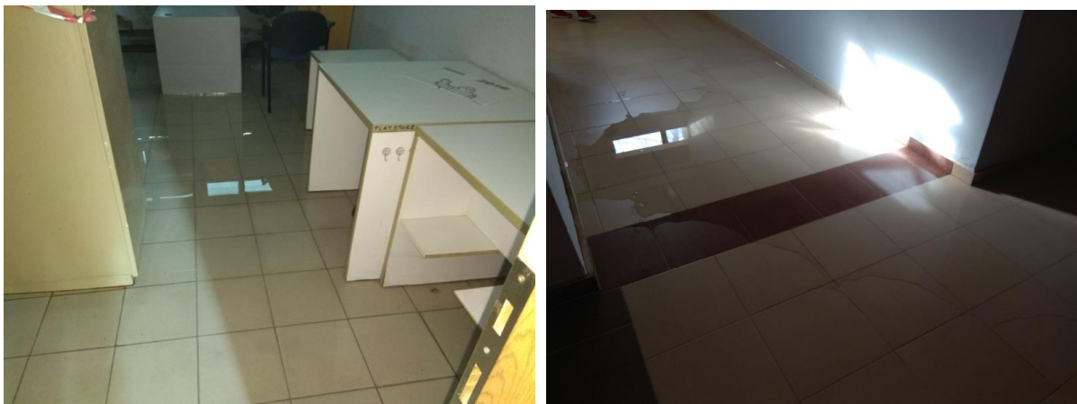
Figure 22. Flooded basement of Building C (teaching and storage rooms and areas)
