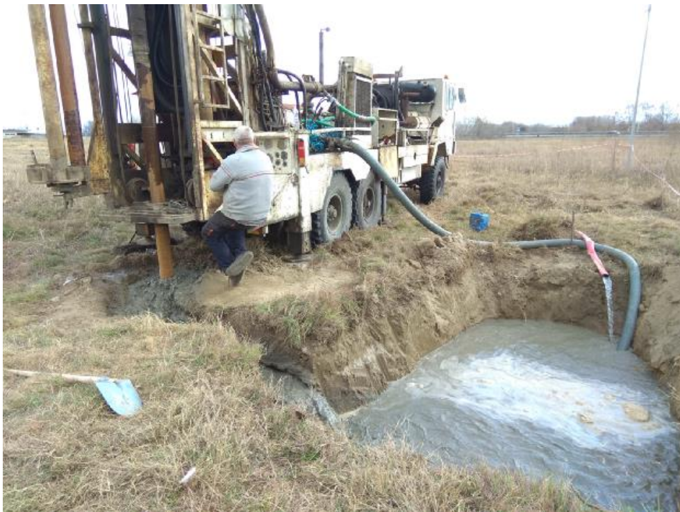
Figure 37. Drilling procedure (the two-fold use of the excavation to provide water and accept the drilling materials can be observed)
