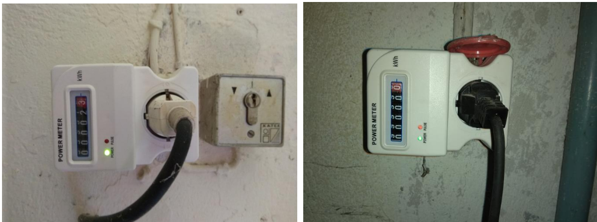
Figure 20. Installation of analogue power consumption measurement devices in the basement of Building B (Pump B1 and Pump B2, photo taken on 17/05/2019)
