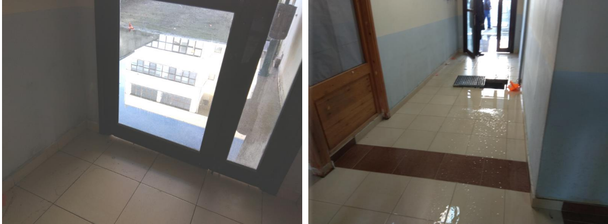
Figure 21. Flooded basement of Building C (ramp area and hall)
