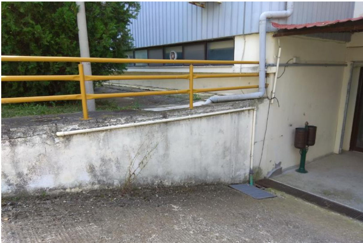
Figure 8. Water pump C2 (Building C) at the base of a ramp. The pumped water is currently driven to the rainwater sewer system.
