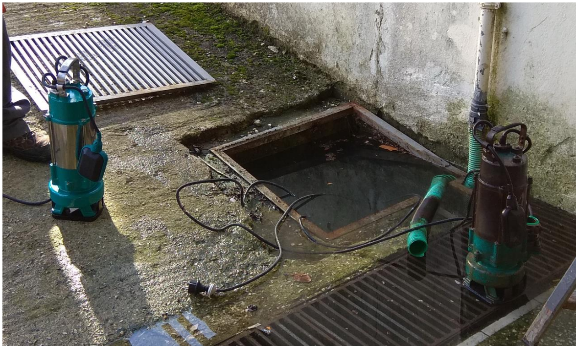
Figure 10. Condition of used and new water pumps (C2) during replacement with same model/type
