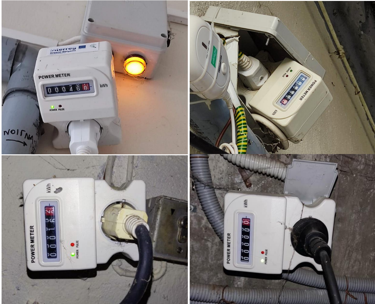
Figure 7. Power consumption measurements of existing water pumps in a) Building C (Pump C1 on the top-left and Pump C2 on the top-right) and (b) Building B (Pump B3 on the bottom-left and Pump B1 on the bottom-right), (photos taken on 11/02/2022).
