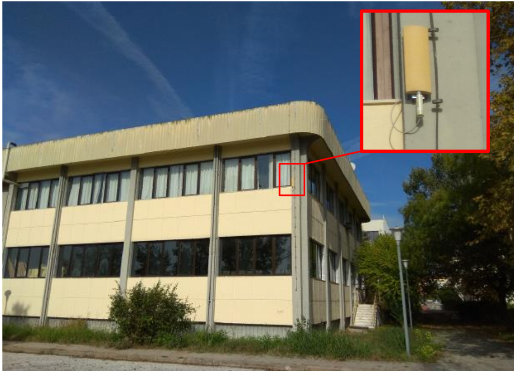
Figure 46. Installation of access point with external antenna to create a new WiFi network for the aquifer monitoring device connectivity
