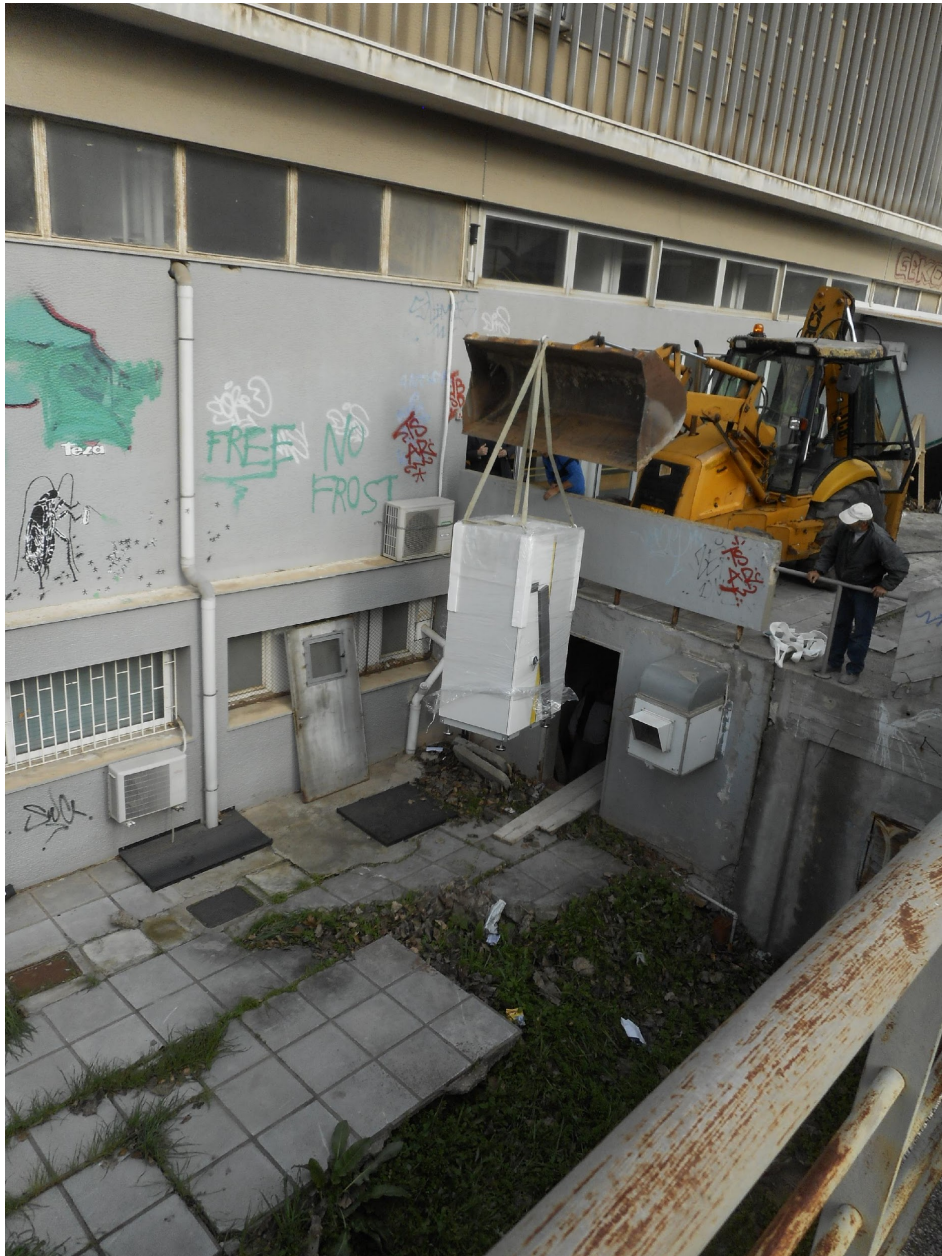
Figure 19. How the heat pumps were able to be transferred inside the building
