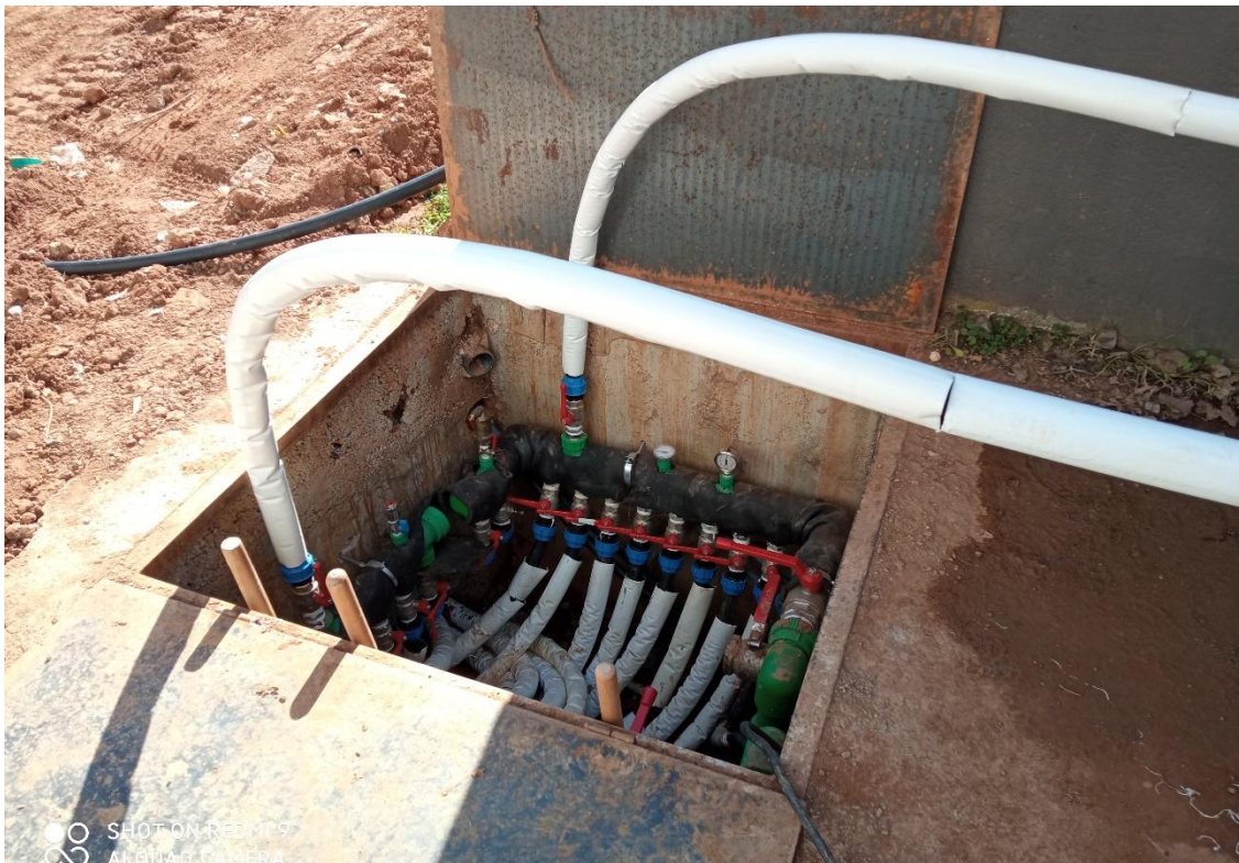
Figure 30. The central manhole of the geothermal heat exchanger
