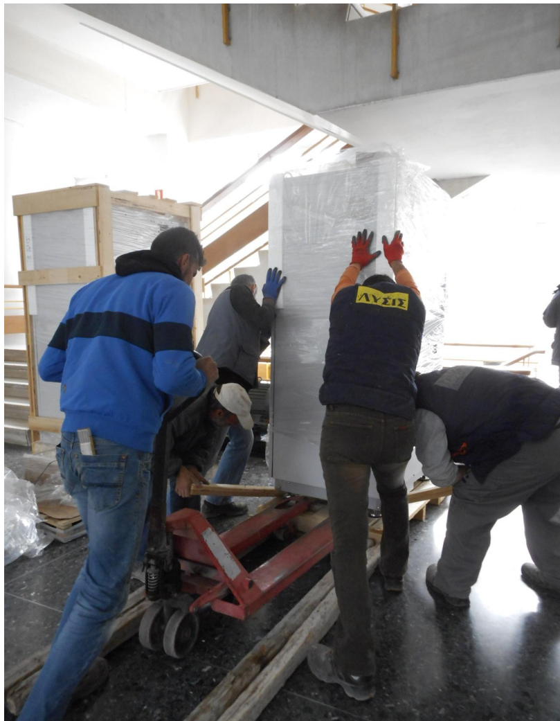
Figure 18. Transporting the heat pumps at the ground floor of the building of Hydraulics
