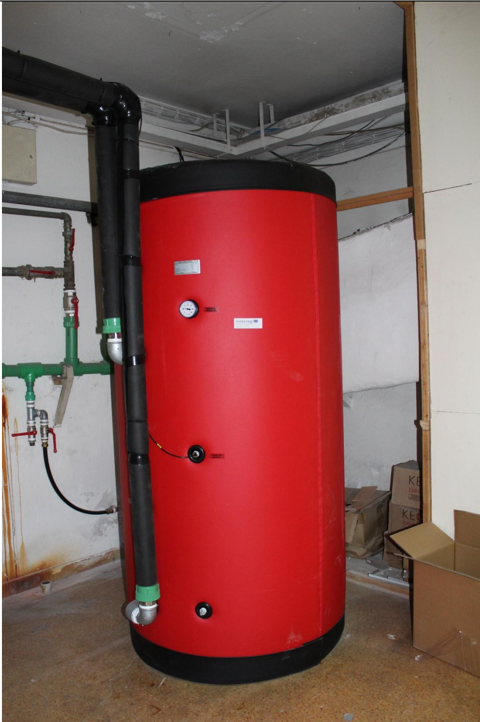
Figure 11. The expansion tank
