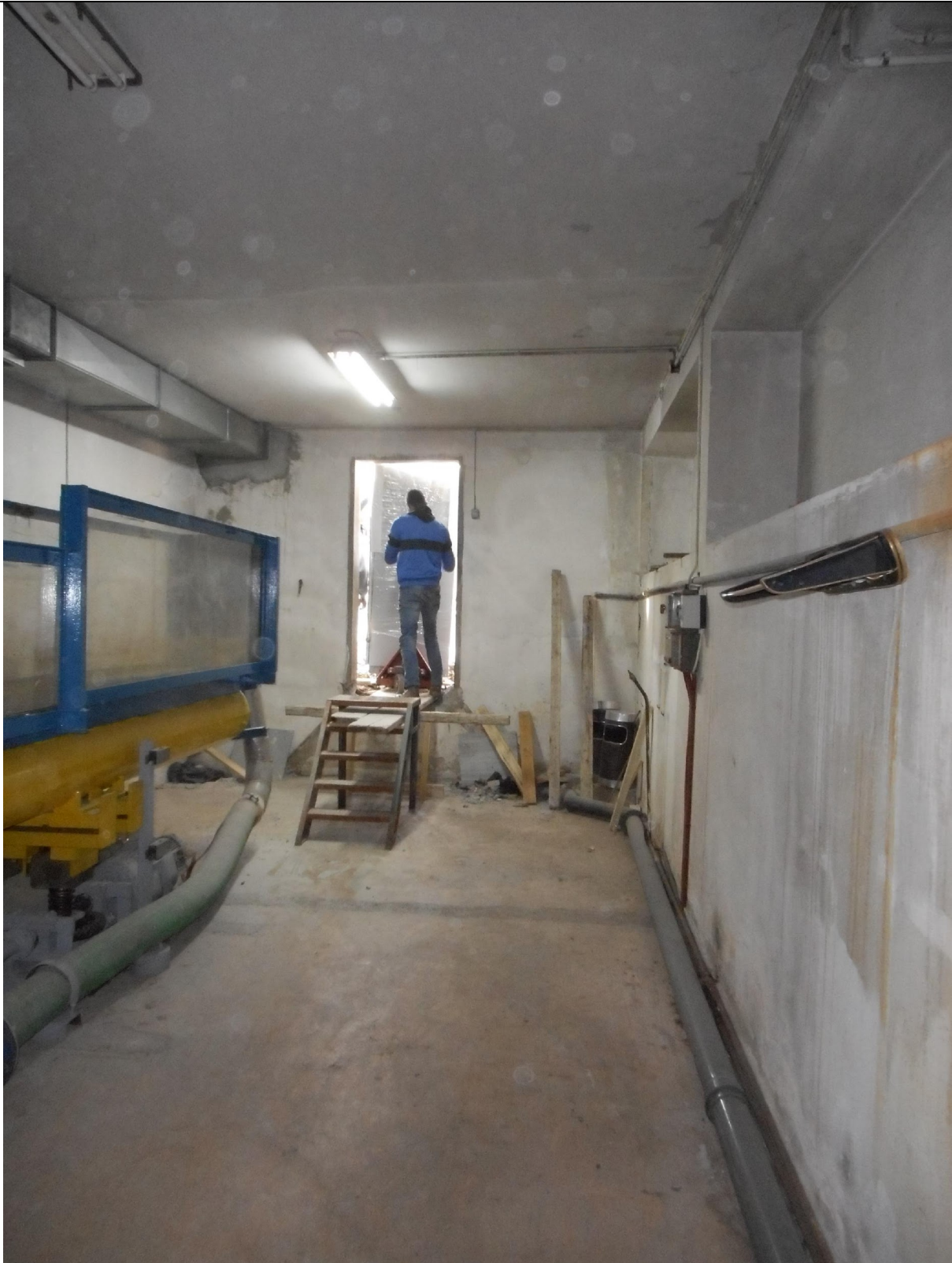
Figure 22. Transferring the heat pump inside the building (as seen from the inside)
