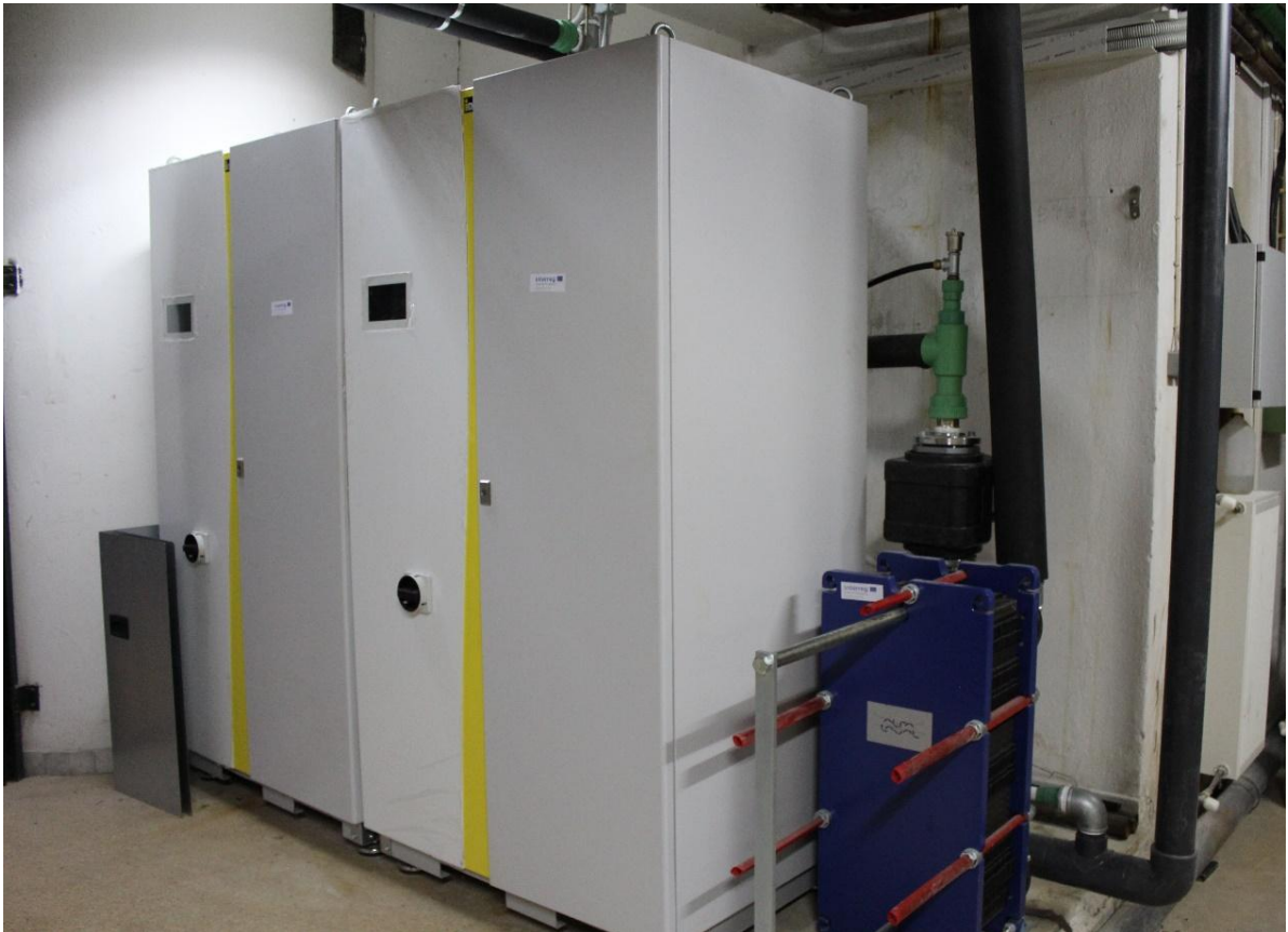
Figure 7. The heat exchanger (blue piece) and the heat pumps (grey)
