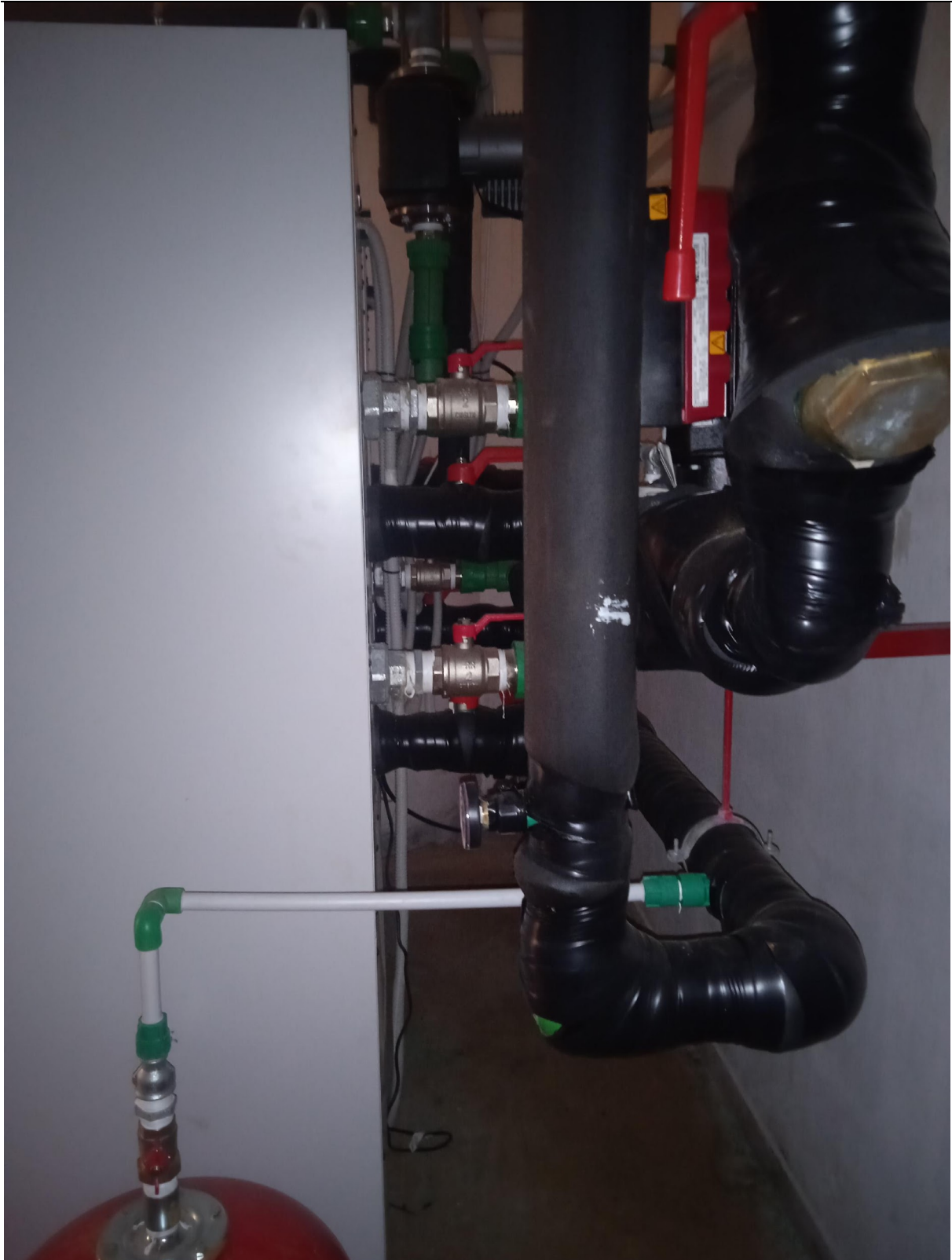
Figure 10. The pipe system behind the heat pumps
