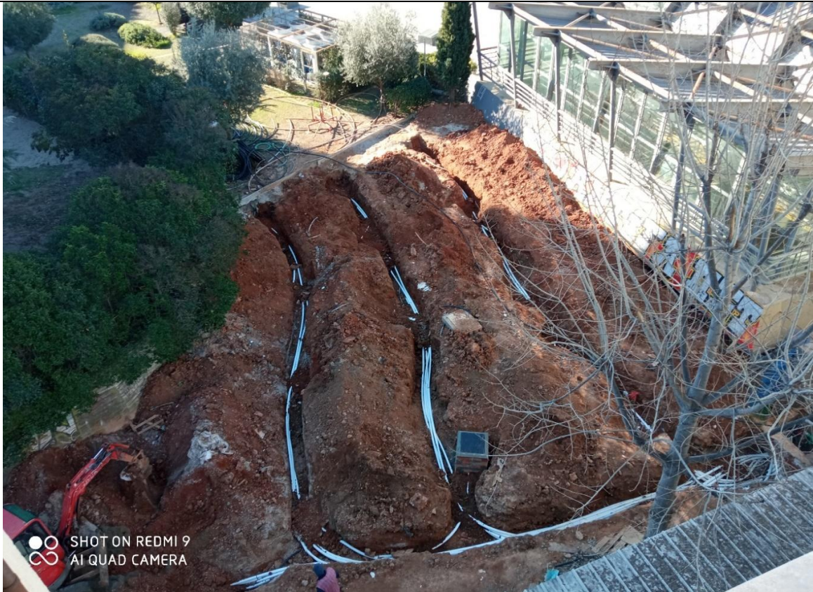
Figure 29. The pipe network that connects the heads of the geo-heat exchanger boreholes
