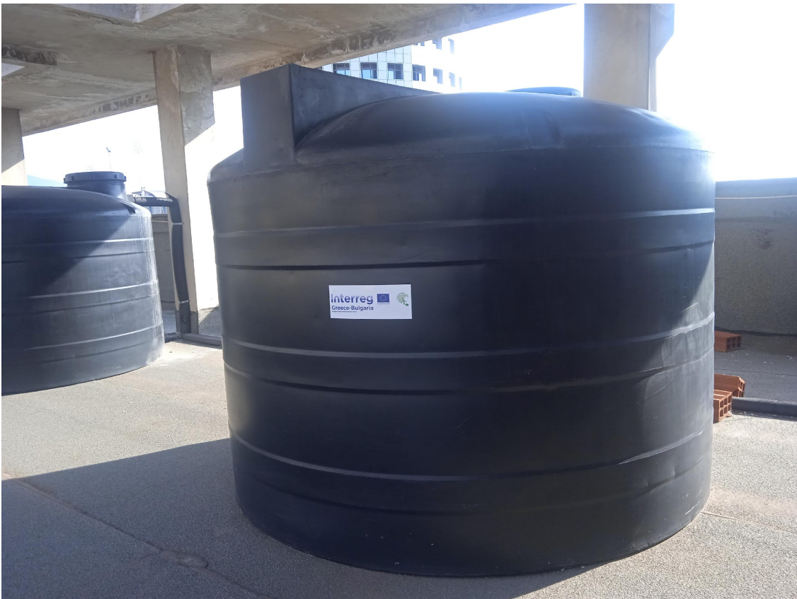
Figure 13. The water tanks (b)
