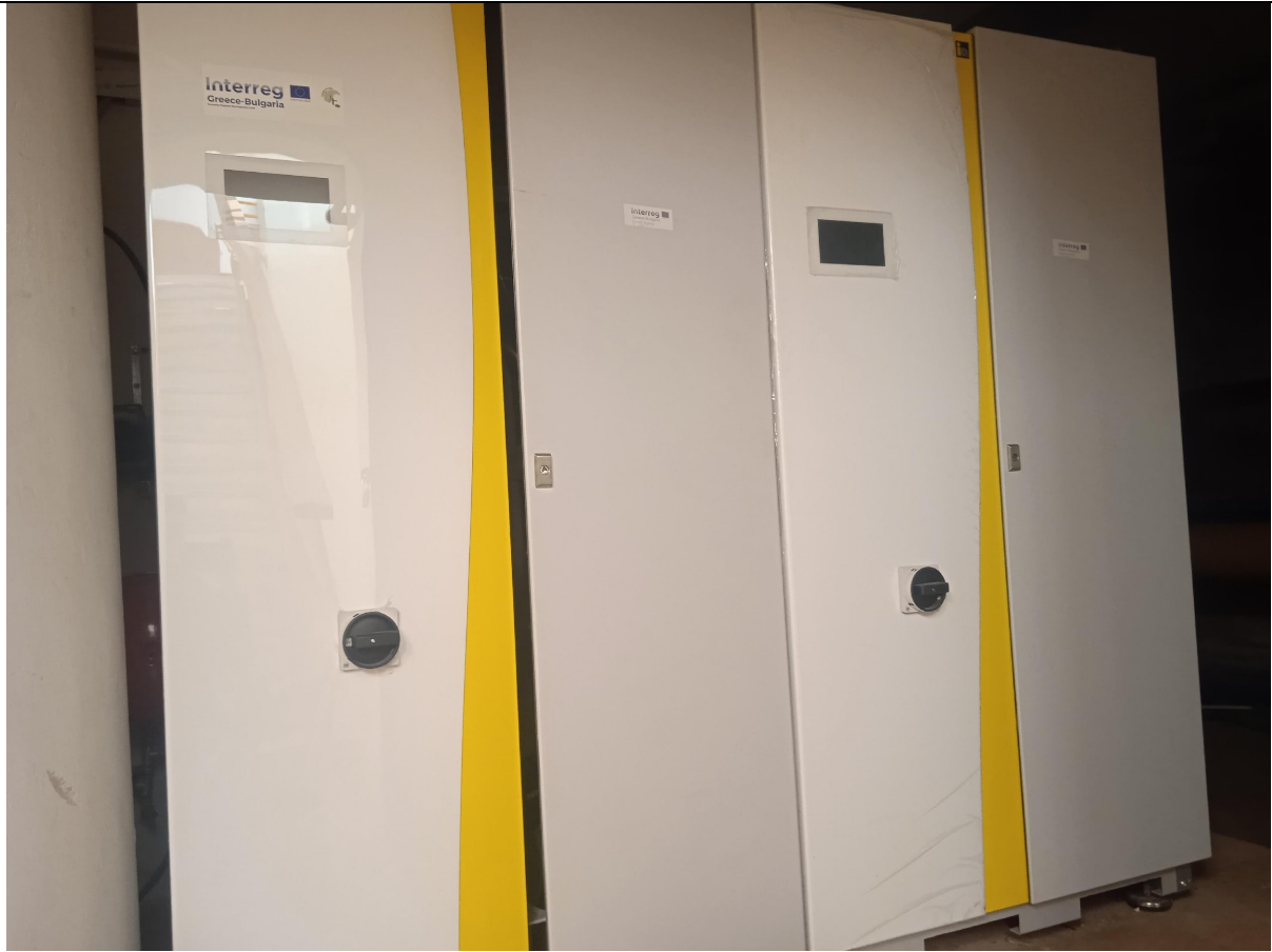
Figure 8. The heat pumps
