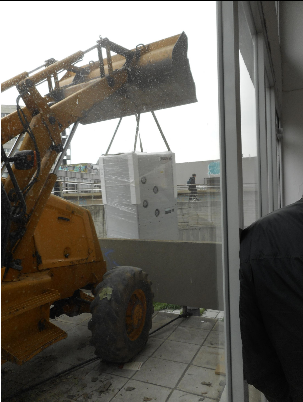
Figure 20. From the successful attempt to place the heat pumps inside the building
