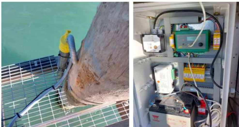
Figure 11. Bocca Scanno station.
