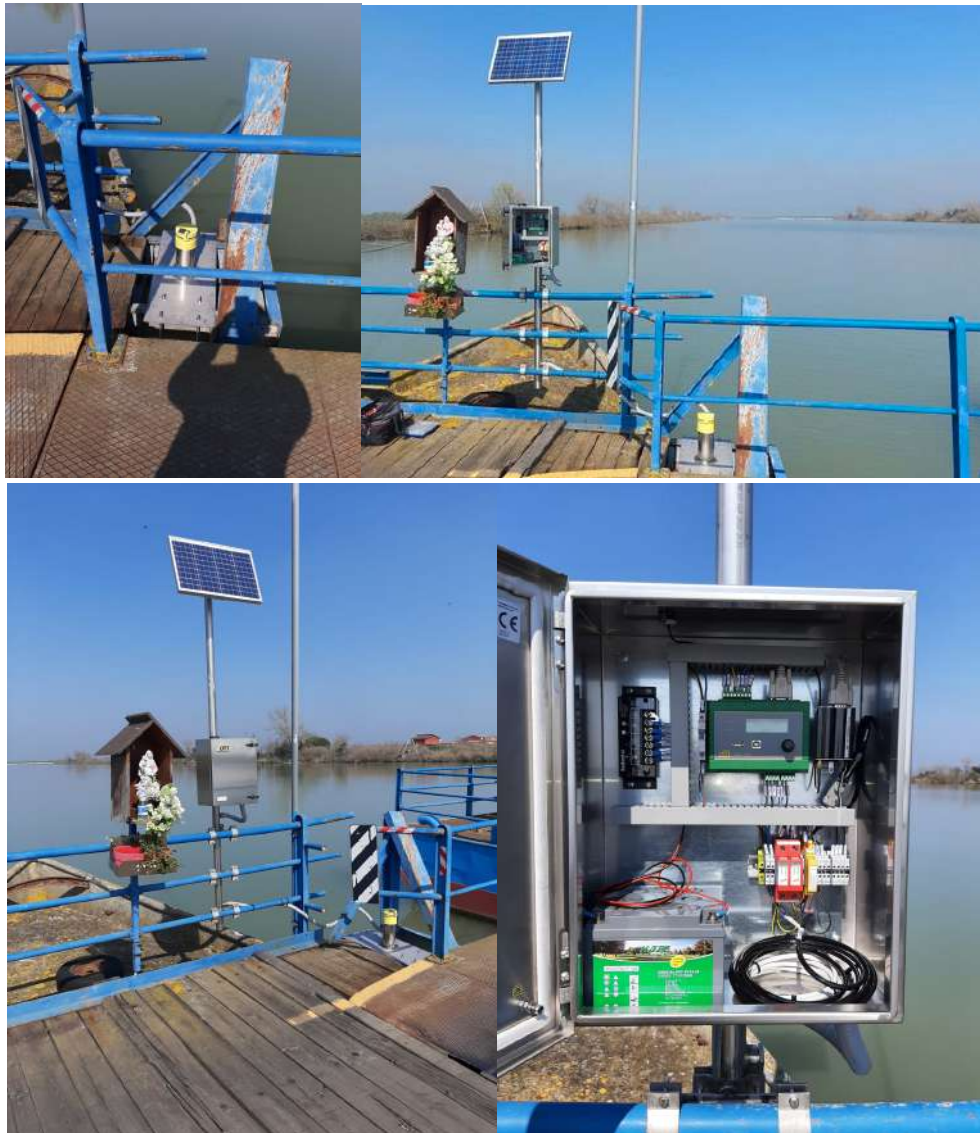
Figure 7. Multiparameter station installed at Po di Goro Location
