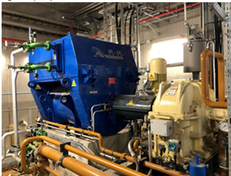
Figure 2 IndaChlor's steam turbine of 0,9MWe
