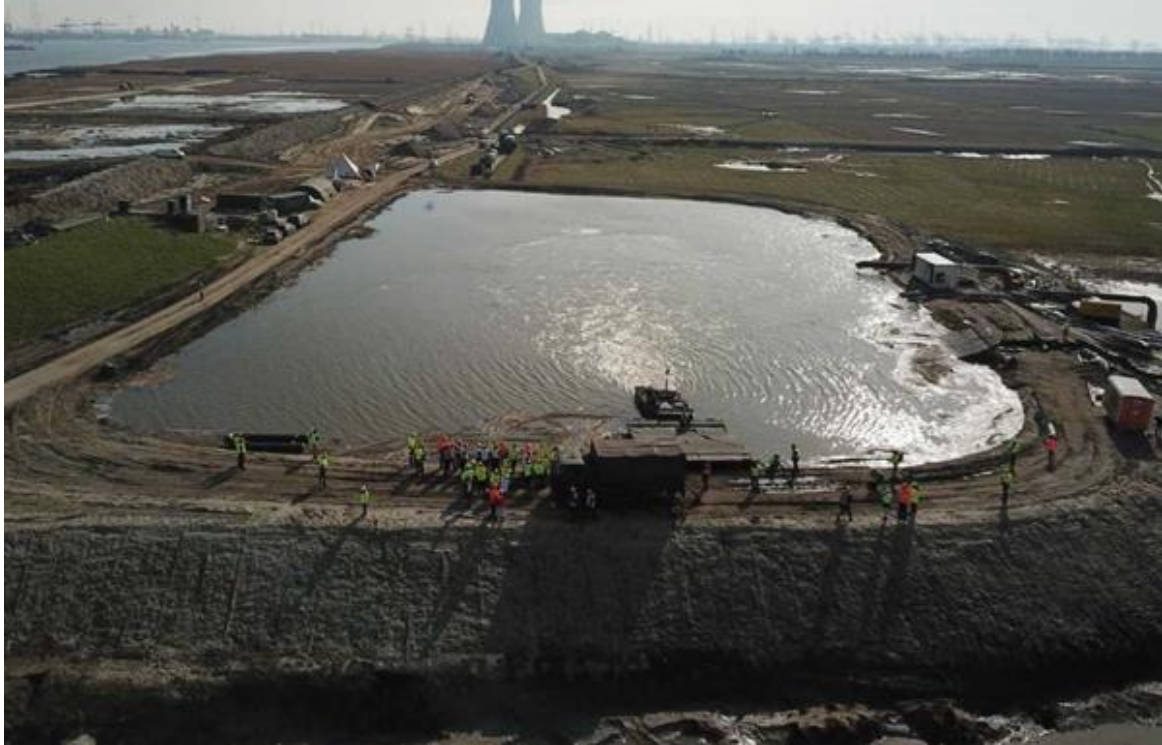
Figure 19 The Hedwigepool (test basin) in the Hedwigepolder, purposely built for emergency response research (mobile barriers and BresDefender), March 2022.
