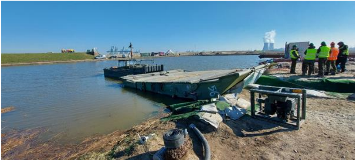
Figure 20 Deployment of the BresDefender emergency response method at an artificial breach in a Hedwigepool levee, March 2022.
