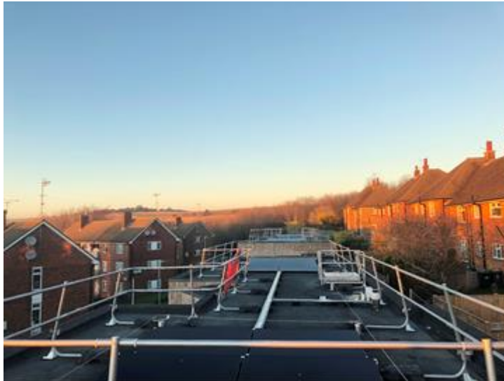
Buckley Close, Brighton with solar installation
