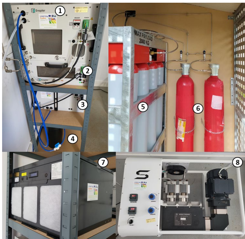
Figure 29: Electrolyzer (1), dryer (2), water tank module (3), water purification system (4), high-pressure hydrogen tank (5), hydrogen buffer tank (6), PEM fuel cell (7) and hydrogen compressor (8).
