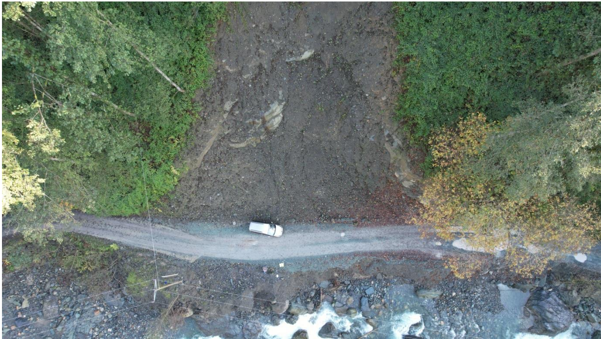
Figure 1. A landslide photo next to a forest road caused by unsupported removal of toe and absence of supporting side wall (photo by Mehmet YAVUZ)
