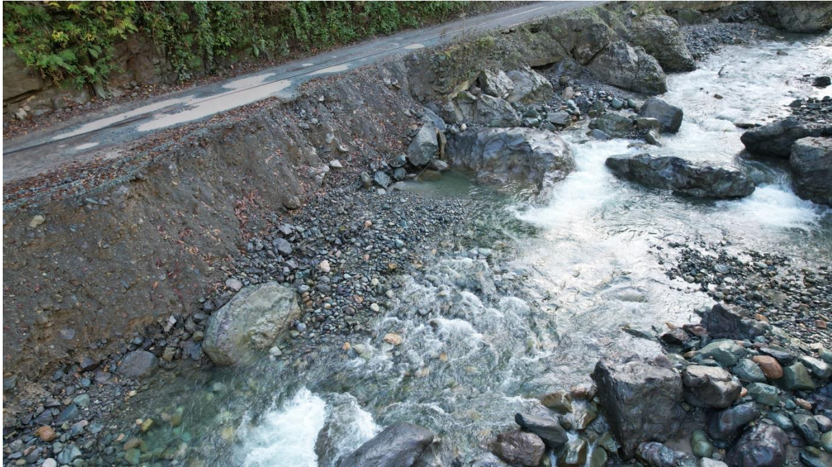
Figure 2. A streambank erosion that threatens the nearby paved road in the Kamilet Valley, Arhavi, Turkey (Photo by M.Yavuz 2021)
