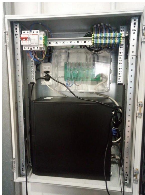
Figure 21: Real-time monitoring system installed setup
