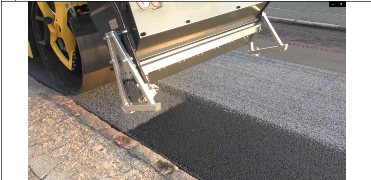
Figure 6: Road roller that spread and compress the granulate into the pavement. Port of Skagen, September 2020.
