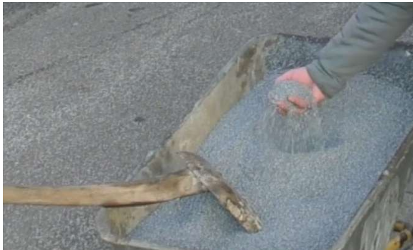
Figure 3: \text{TiO}_2 concrete stone material ready to be compacted into a asphalt pavement.
