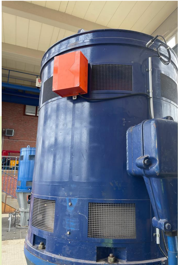
Figure 41. Location of the port's pumping station (left) and the box containing the so called Sensorphone , that detects and records pump activities (right).
