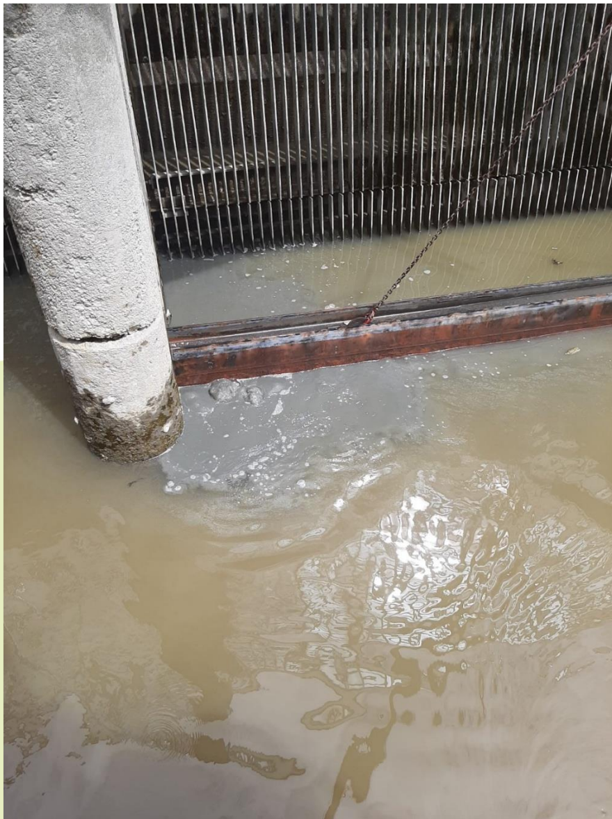
Figure 10. Panel board used as a sediment barrier in the inlet area of Pump 1 at the port's pumping station for the field test.
