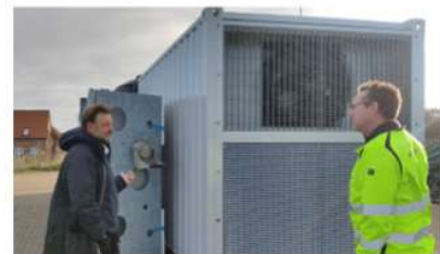
The transformer and inverter technology is packed in two 20" containers
