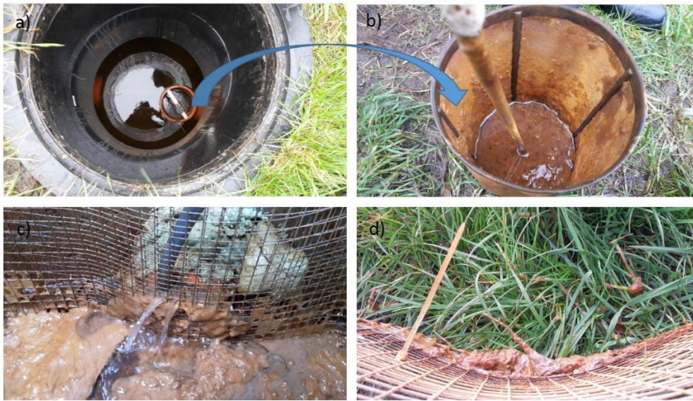
Figure 13 The input of amorphous organic matter via the drain water leads to clogging of the screen filter in the pre-filter (b) and the wire filters in the inlet of the P filter (c and d), as well as the ICS. As a result, the water level in the pre-filter rises and causes overflow of the screen filter and the input of even more amorphous organic matter.
