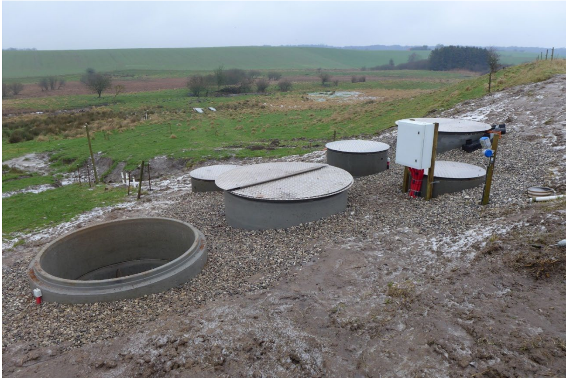
Figure 2 Drainage P-filter system near Odder, Denmark.
