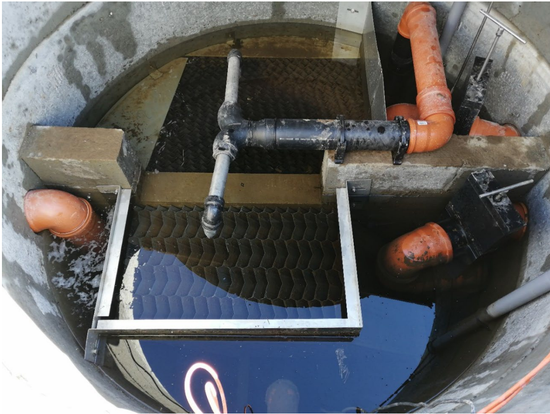
Figure 3 Well housing Hydroseparator™ for retaining drainage sediment and particulate P.
