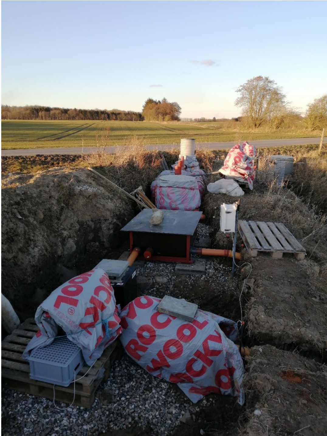
Figure 2 Drainage P-filter system near Odder, Denmark.
