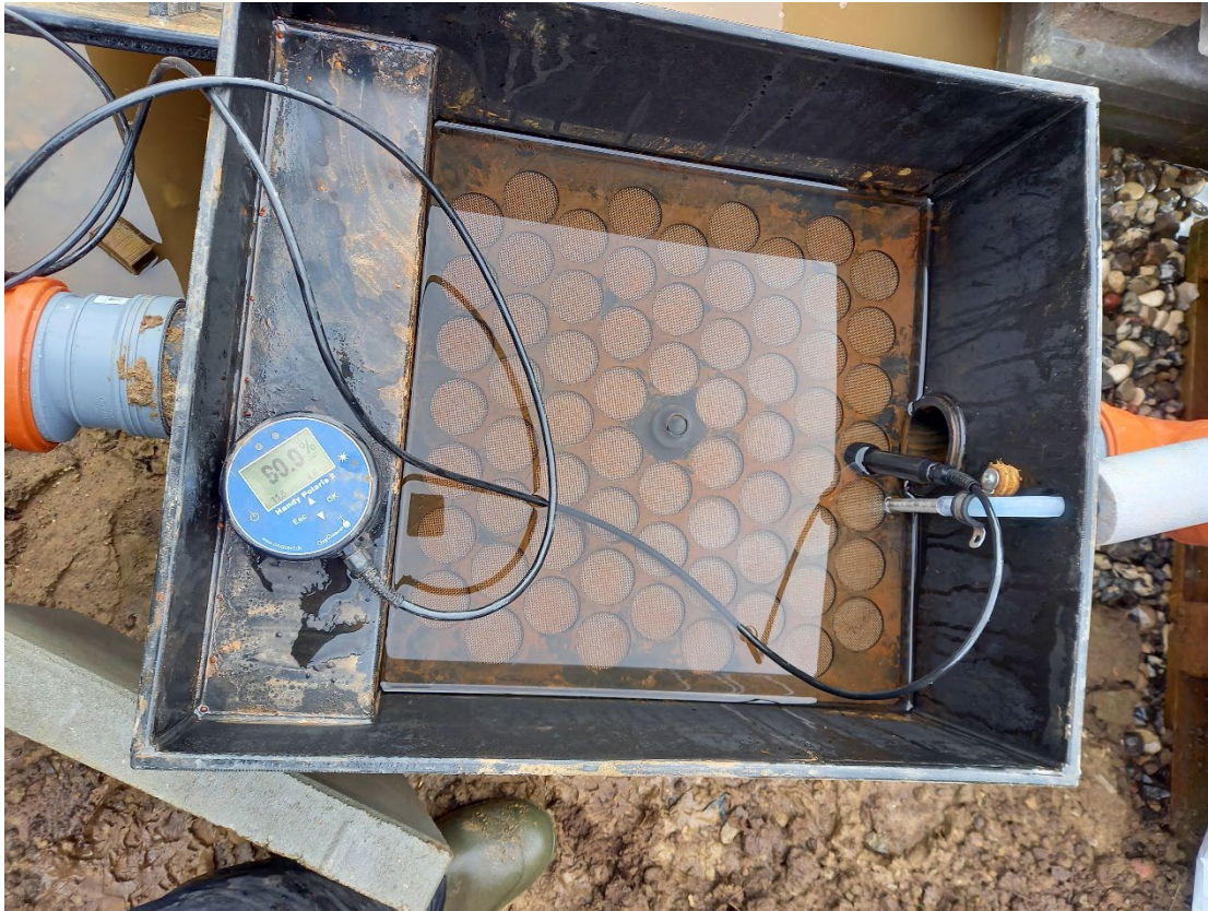
Figure 5 Filter box with reactive ICS filter
