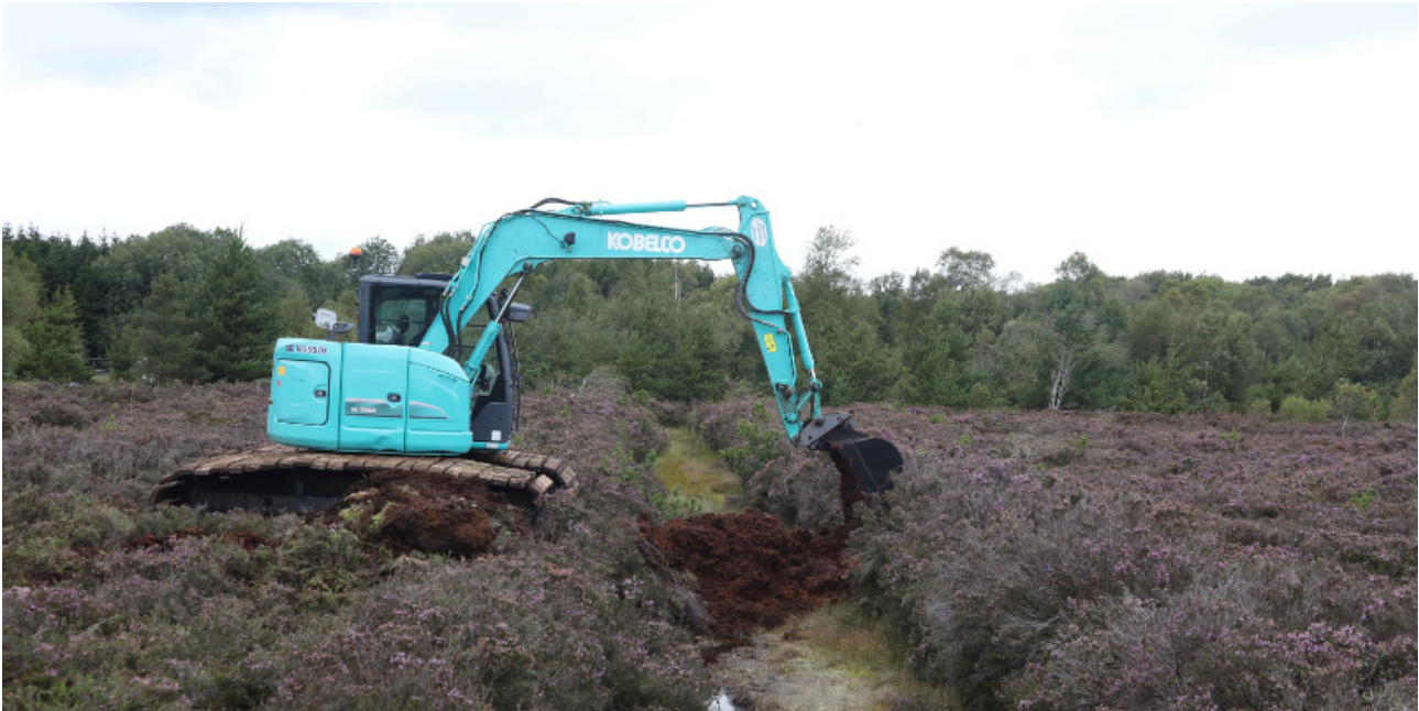
Figure 9: Drain blocking at pilot site (Photo: Eugene Dunbar)
