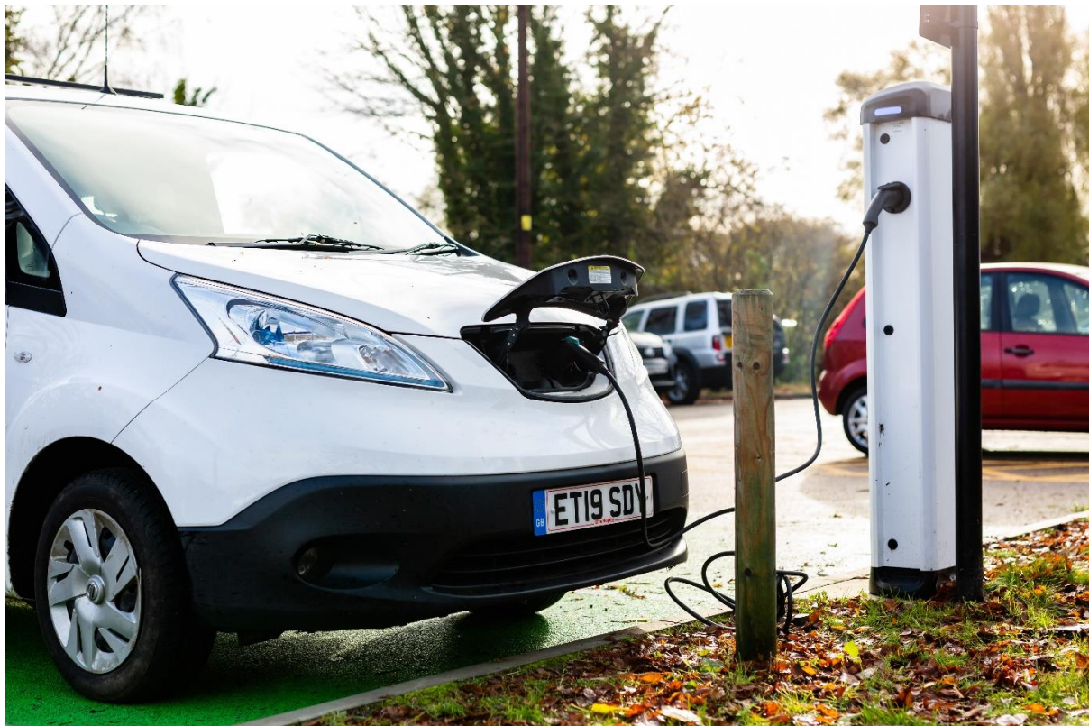
Figure 12: Electric Charging Point
