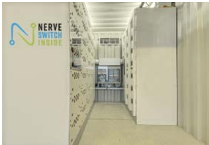
Figure 6.2.1 Containerised battery system with Nerve Switch System hardware. Source Nerve Switch System ApS.
