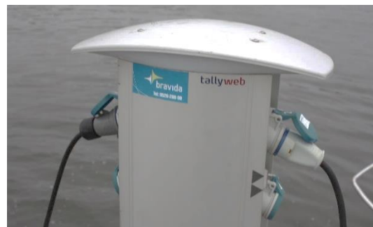
Figure 8. TallyWeb charging infrastructure for onshore power demands.
