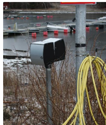
Figure 13 – Simple electrical outlets at shore in Hålkedalen
