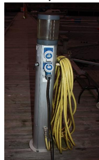
Figure 11 – Dock lights with electrical connection possibilities at Myren leisure boat docks
