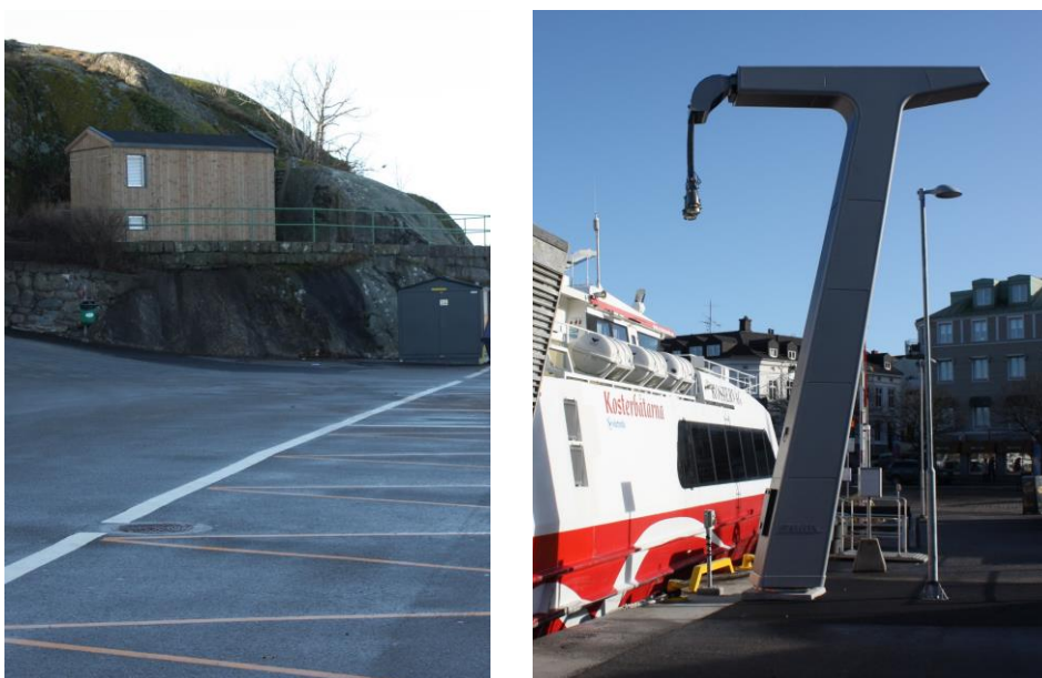
Figure 25. Charging infrastructure for the Kostervåg in Strömstad's north harbour – transformer station on the left and charging tower on the right
