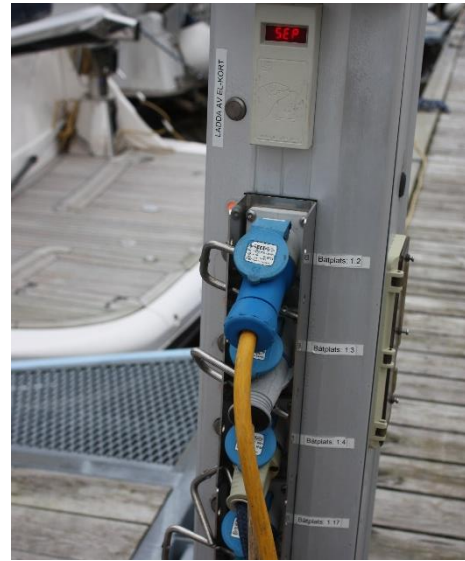
Figure 5. Electrical outlets for use by recreational boaters at Strömstad Marina AB.
