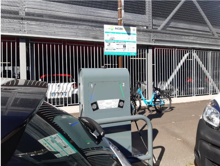
Figure 14 June 2021 : Informative Panel and charging station at Mobipoint "Dreux Gare"
