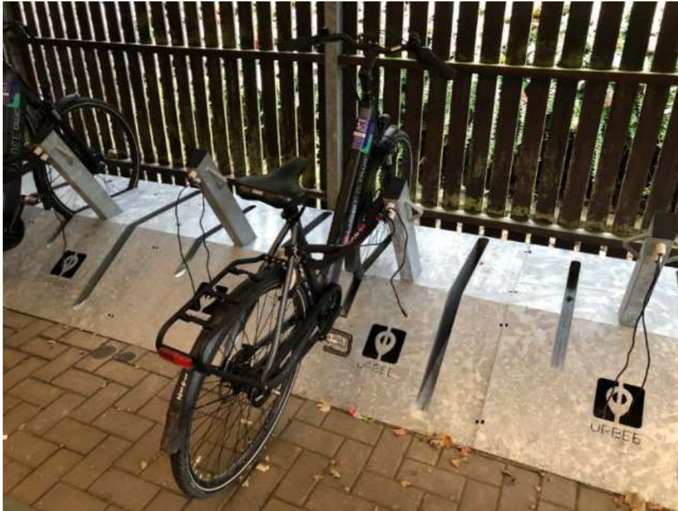
Figure 86 November 2021 – Charging infrastructure e-bikes at eHub Gasthuisberg
