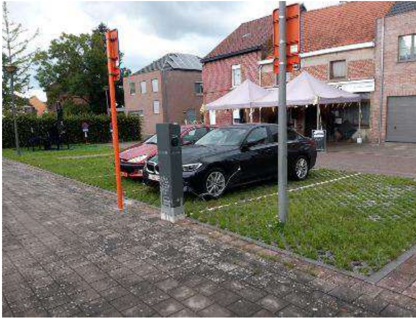
Figure 79 Charging infrastructure at eHub Egenhoven Centrum
