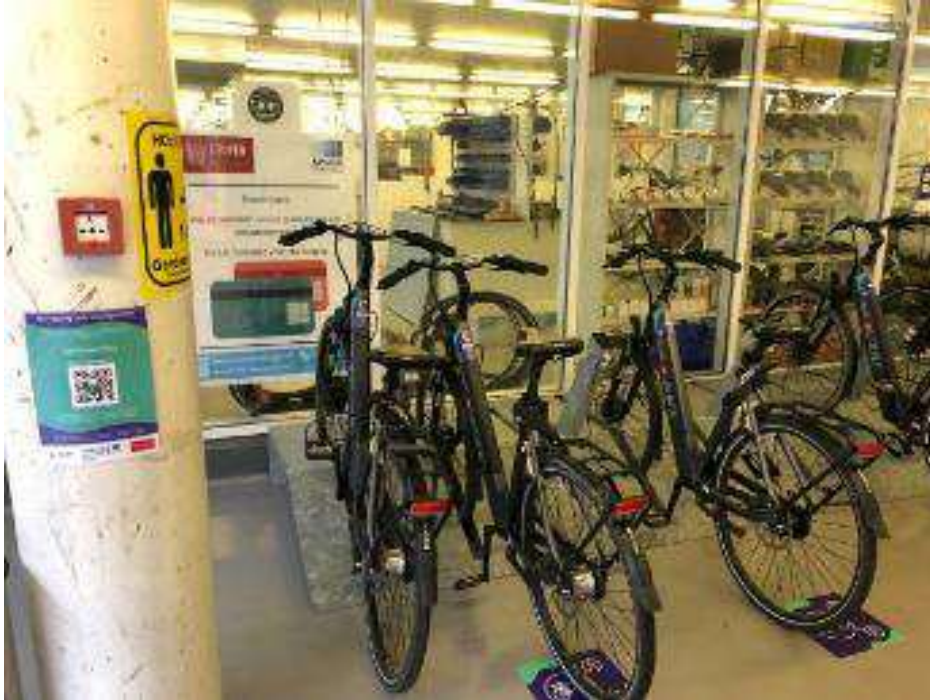
Figure 46 November 2021 – Charging infrastructure e-bikes at eHub Rector De Somerplein
