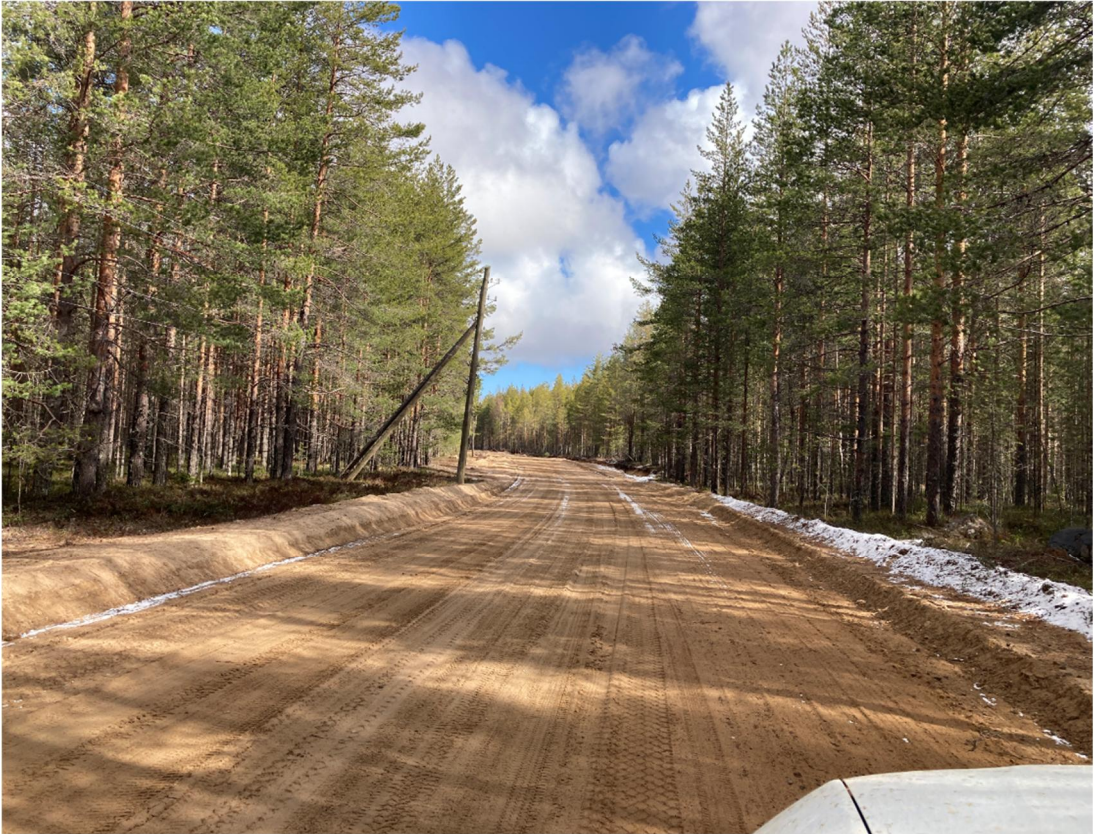
Picture. Current Sumposad - Kolehma regional road in the Republic of Karelia (Photo: Vyacheslav Lyapin, Domer PK)
