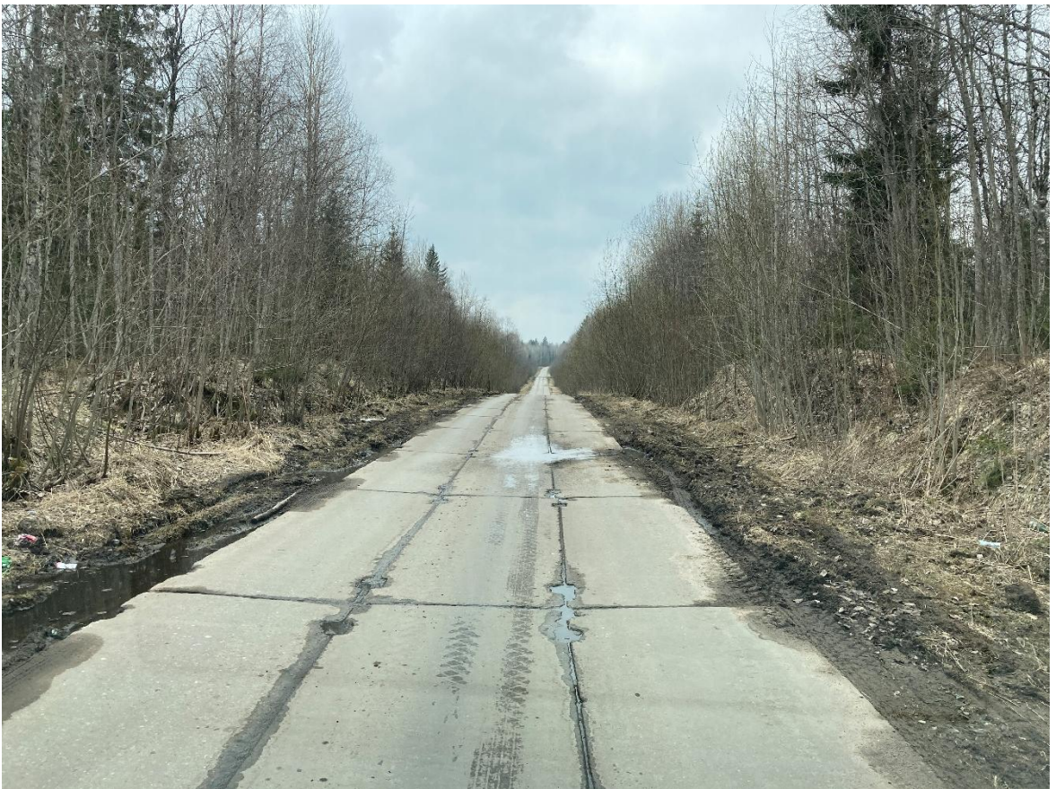
Picture. Current regional road Kyanda – Rikasikha near Rikasikha (concrete road) (Photo: Vyacheslav Lyapin, Domer PK)
