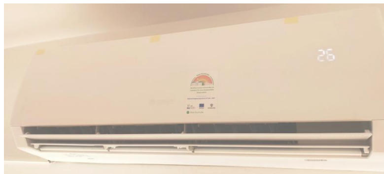
Figure 11: High performance air conditioning units
