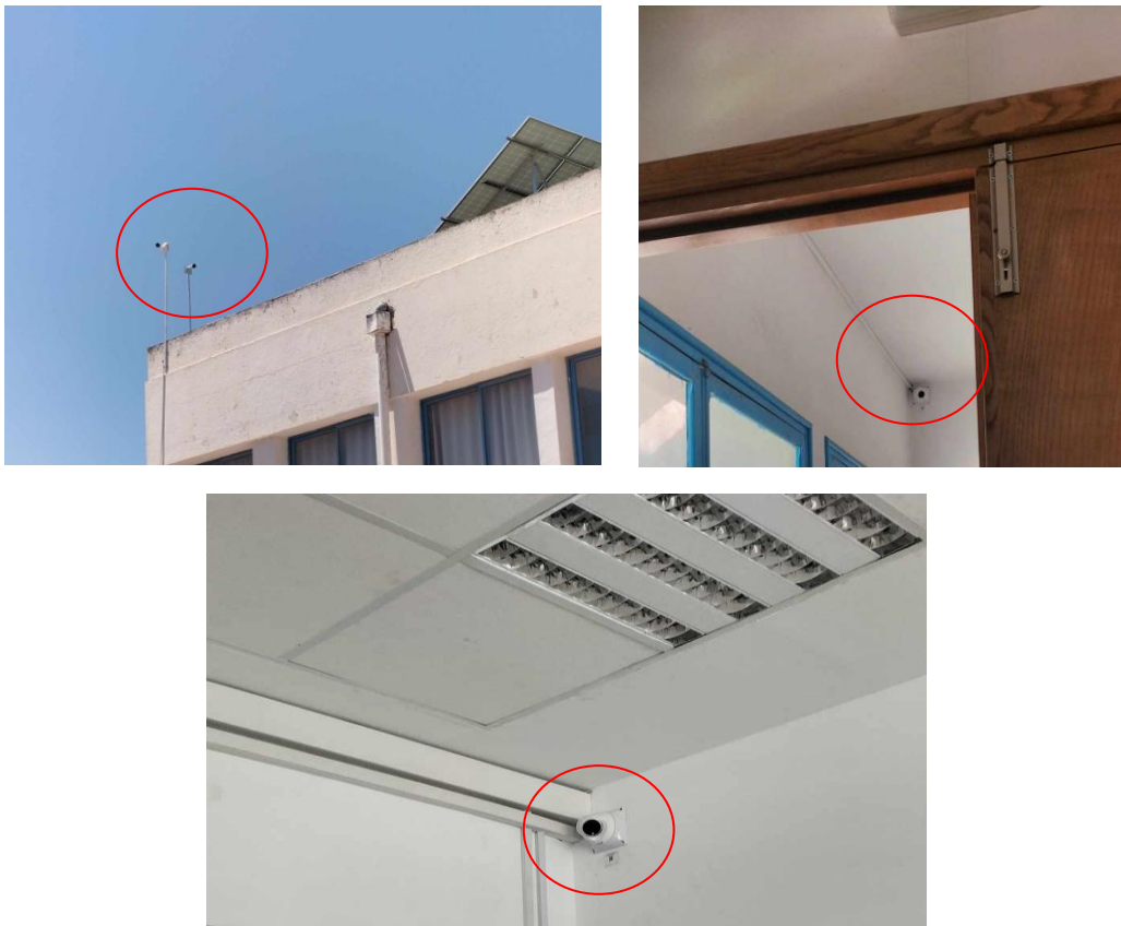
Figure 12: Surveillance and security cameras
