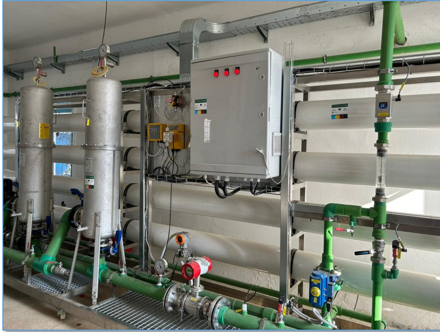
Photograph 5. Desalination plants in Tunisia, control panel
