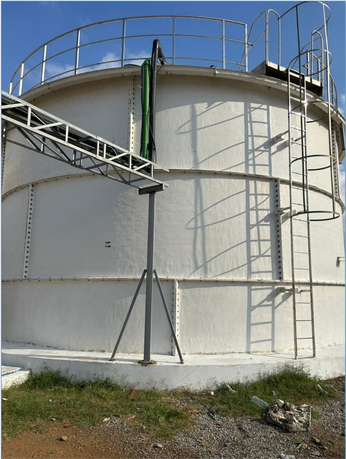
Photograph 7. Water storage tank for desalinated water.
