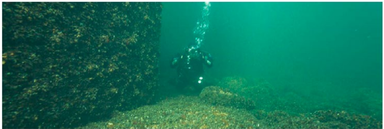
Figure 11. Mussels colonizing the Öresund bridge (Bucefalos project report, Design of full scale blue mussel cultivation site in Öresund)
