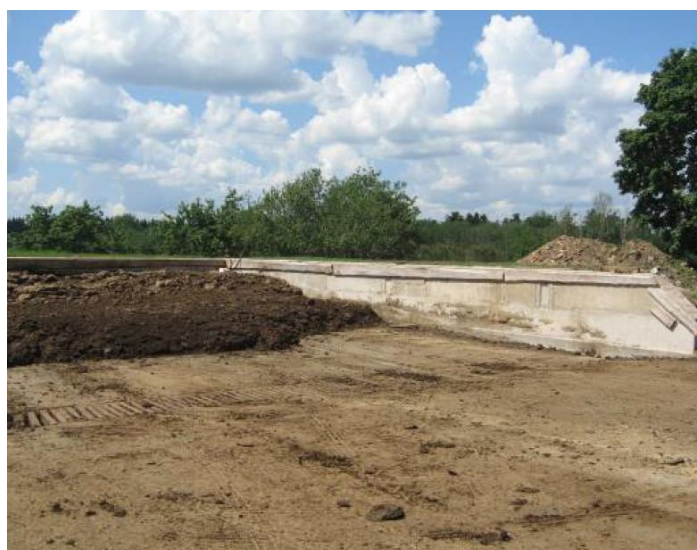
Figure 2-13. Storage for solid manure, concrete platform with walls.
