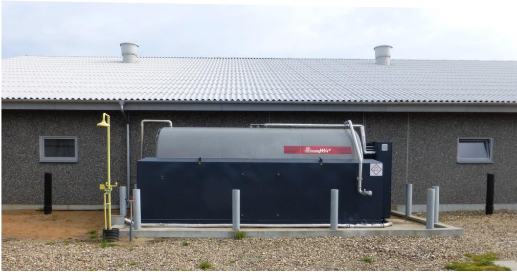
Figure 4.2. Acid tank based on concrete platform outside a pig house.
